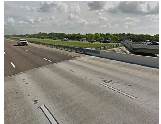
The areas where an asphalt pavement approaches or departs a concrete bridge are susceptible to specific kinds of distress.
