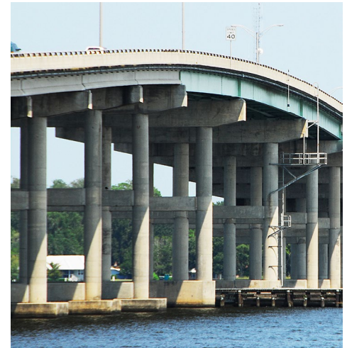
Excessive curing temperatures in large concrete structures can result in cracking and less durability.
