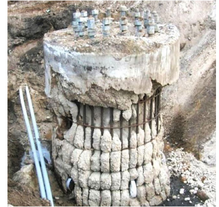
This recovered drilled shaft shows the mattressing effect caused by concrete flowing radially through the reinforcing cage.
