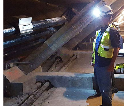
Inside a concrete structure, a worker uses a version of the device developed in this project to examine a post-tensioning tendon.
