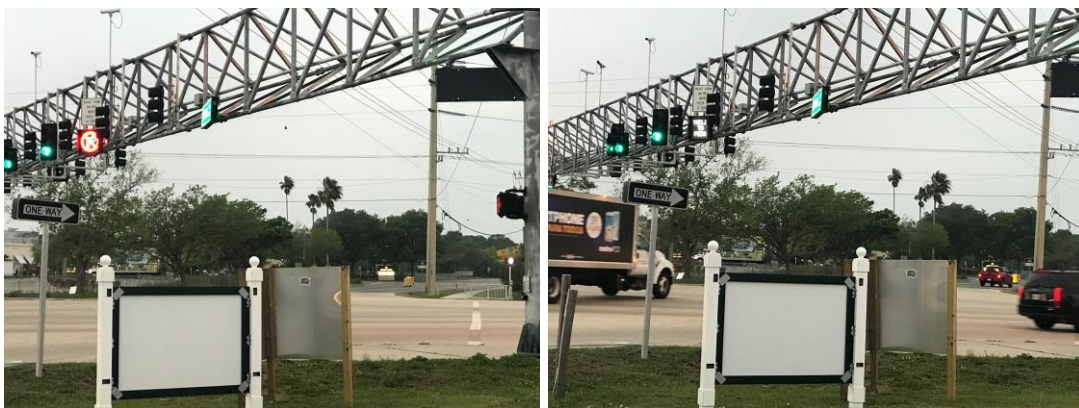
Figure 7-2 Dual blank-out “NO TURN ON RED”/“YIELD TO PEDESTRIANS” sign.
