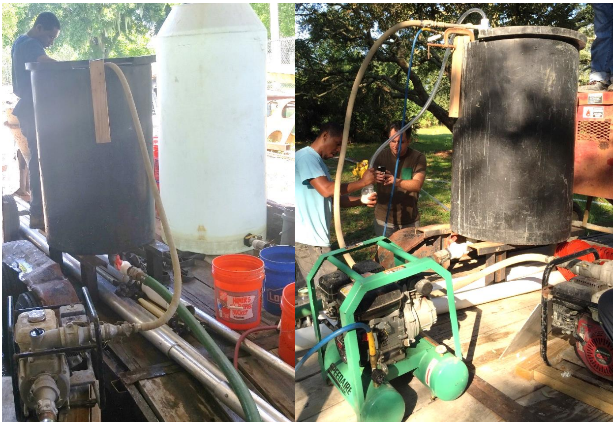
Figure 3.8 Slurry mixing system; re-circulating (left), mixing (right).
