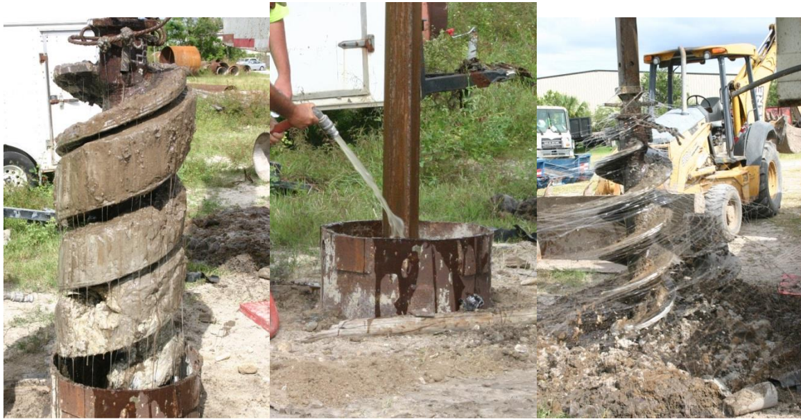
Figure 4.14 Auger extraction (left), slurry replacement (center), and polymer strings during auger spin off (right) of Shaft P0-100.
