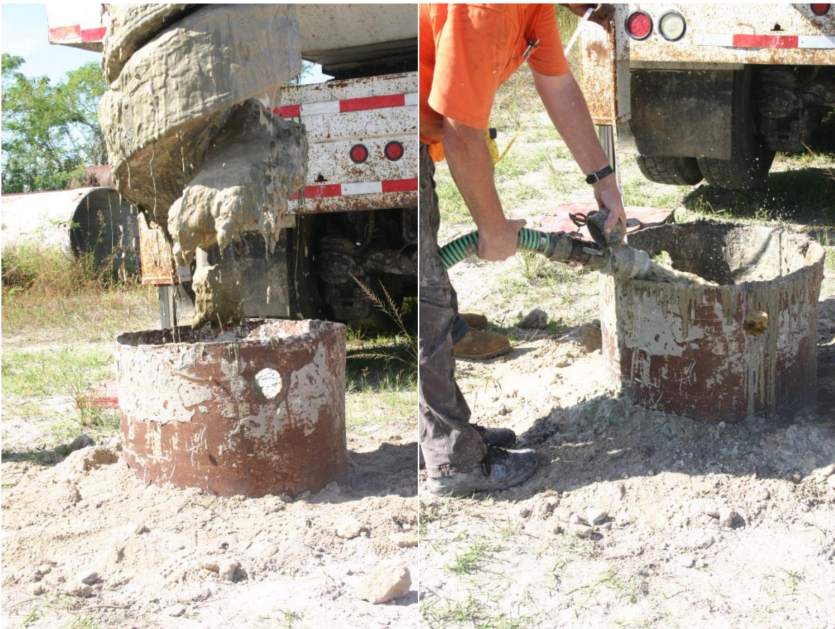
Figure 4.13 Auger extraction (left) and slurry replacement (right) during construction of Shaft B48-40.
