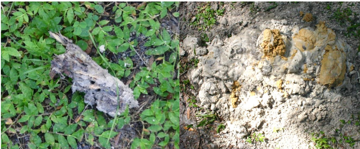
Figure 3.83 Excavation difficulties resulting in reduced shaft length; portion of root (left), clayey-sand soil (right).
