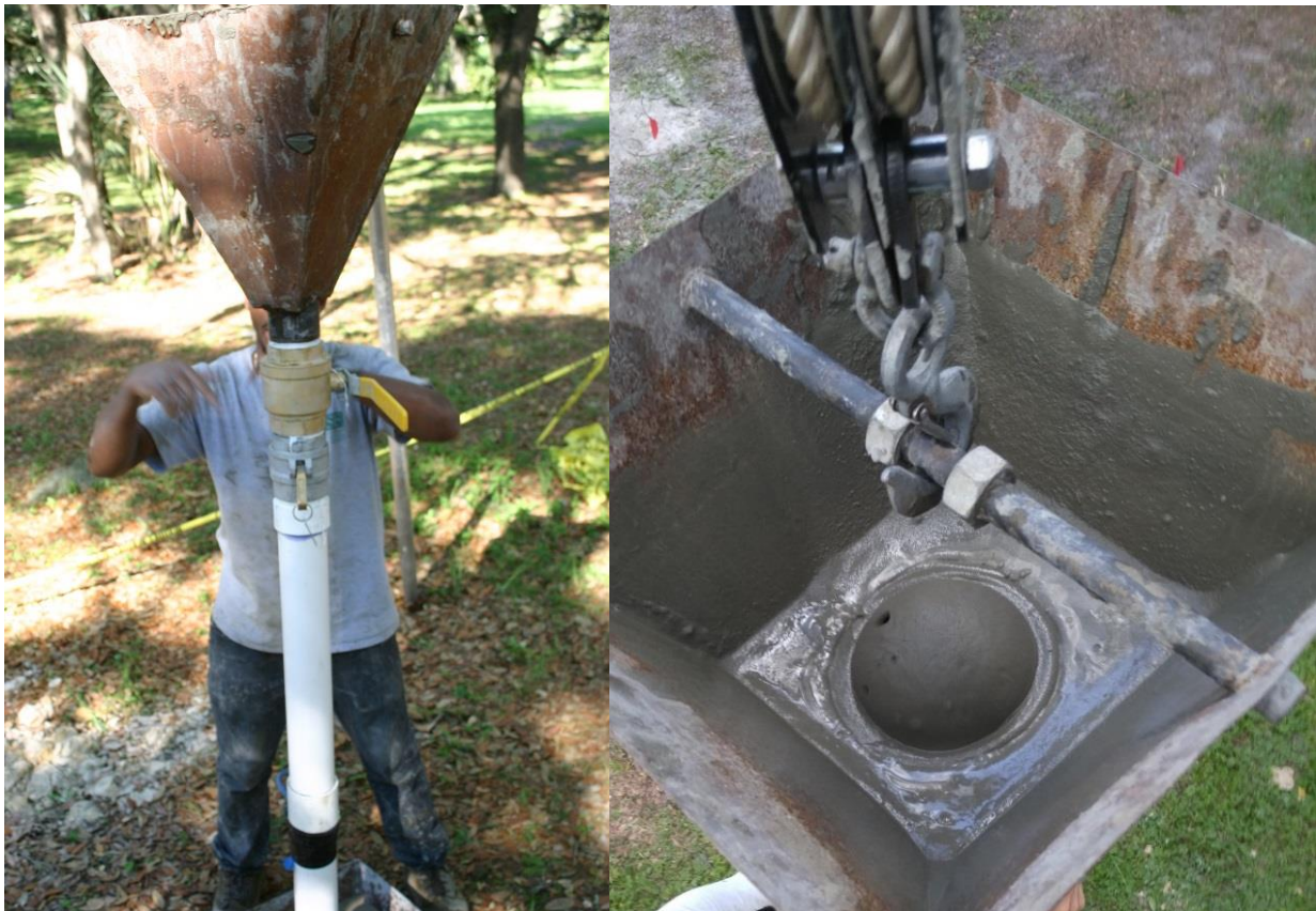
Figure 3.47 Hopper connected to the tremie (left), confirmation of mortar flow into tremie (right).
