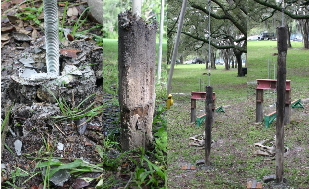
Figure 3.53 Shaft extraction; breaking ground surface, 2ft, 4ft, and 6ft extracted (left to right).
