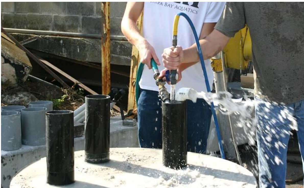
Figure 3.10 Airlift vacuum used to clean up fragments from inside the installed casings.
