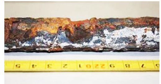
This rebar taken from a piling shows corrosion's effect on reinforcing steel. Corrosion of the steel also damages the piling concrete by expanding and causing the piling concrete to crack.
