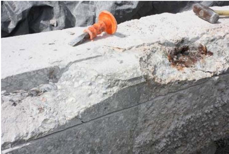
Figure 9. Oxide stains in concrete cover observed during removal of embedded bar.
