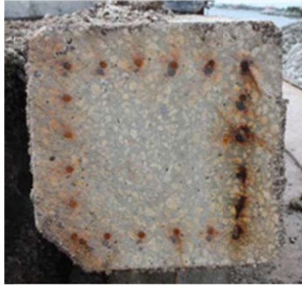
Figure 21. Submerged (i.e., bottom) end of extracted pile, end view. Note that the absolute bottom end of the in-service pile was left in situ and that this pile segment was cut from it.
