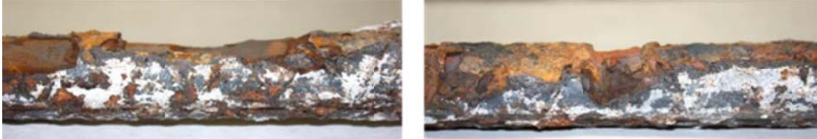
Figure 12. Apparent corrosion-related cross-section loss observed in bar #1.
