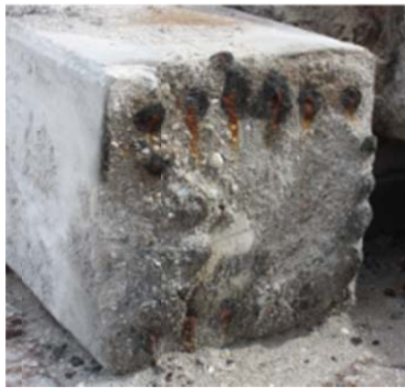
Figure 20. Atmosphere-exposed (i.e., top) end of extracted pile.
