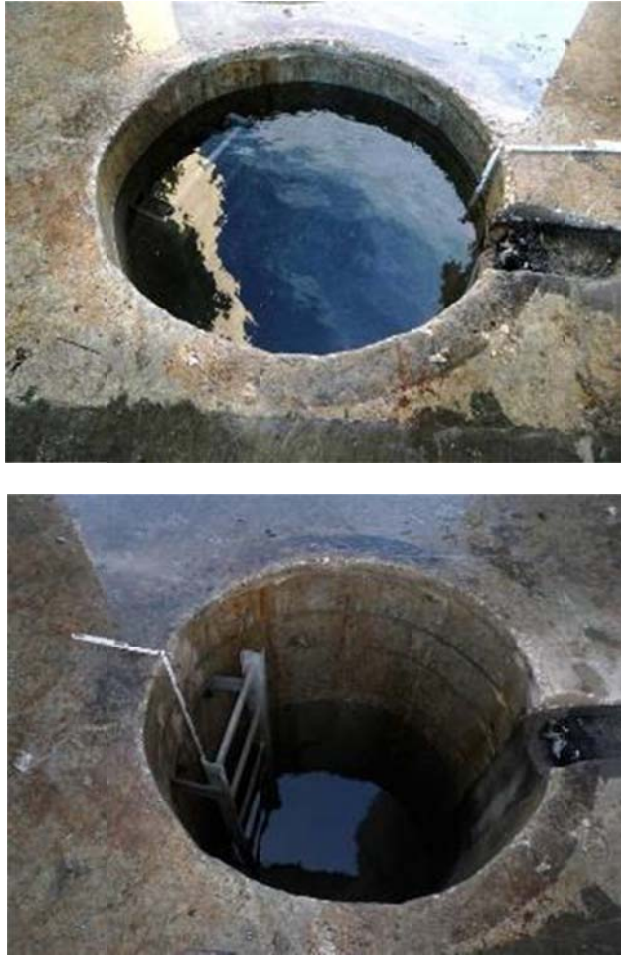
Figure 44. Top: Water level 30 minutes after filling, Pier 112. Bottom: Water level approximately 2 hours after filling, Pier 112.
