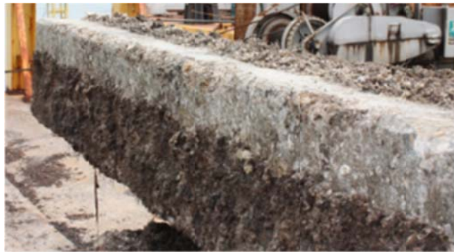
Figure 24. Submerged end of pile selected for autopsy. Note that marine growth has been scraped from the surfaces near the corner to facilitate saw cuts.
