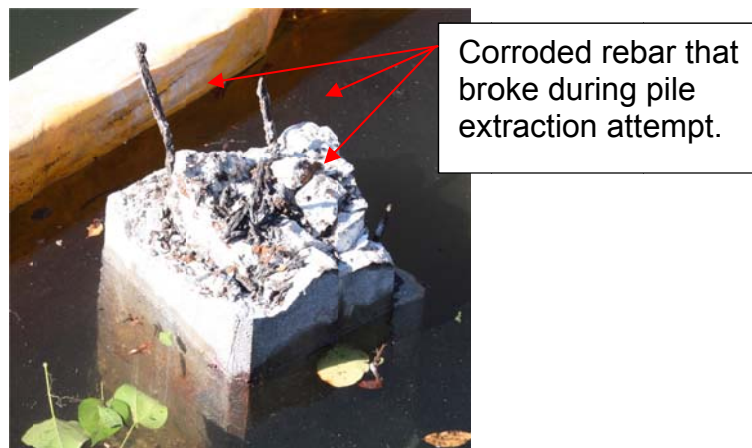
Figure 32. Bottom half of pile left in place as a result of breakage during extraction attempt. Visible rebar corrosion and section loss in splash zone.
