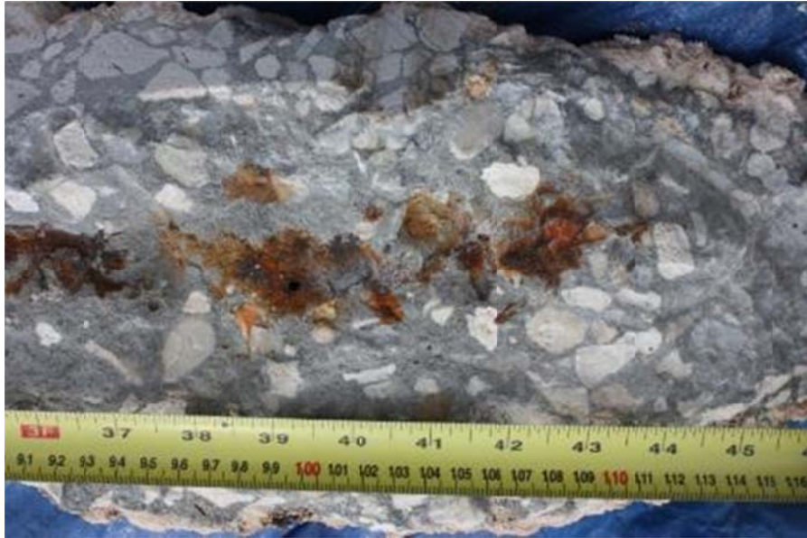
Figure 7. Rebar rust trace on portion of concrete removed from Pile #1. Tape measure indicates distance from bottom of pile.
