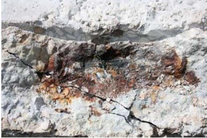
Figure 10. Close-up view of oxide stains in concrete cover observed during removal of embedded bar. Note that a small portion of the bar itself can be seen in the center of the photo.
