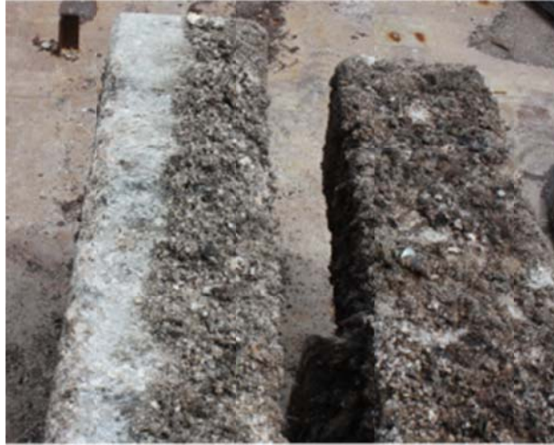
Figure 23. Marine growth on the submerged regions of two piles. Note that some growth has been removed from the surface of the pile on the left in preparation for autopsy/saw cutting.
