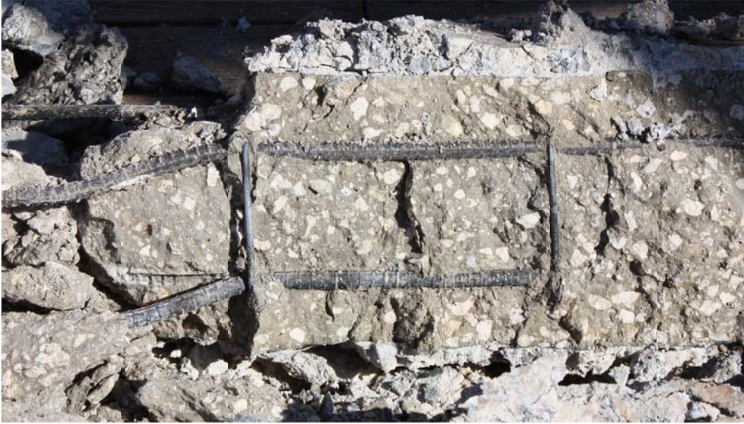
Figure 33. Corrosion-free steel in much of the submerged region. Note that pile in photo was lying on its side.
