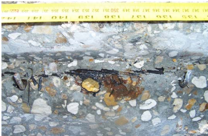
Figure 29 top, middle, bottom. Three different instances of localized corrosion. Note that the measurement datum for the indicated distances was the waterline.
