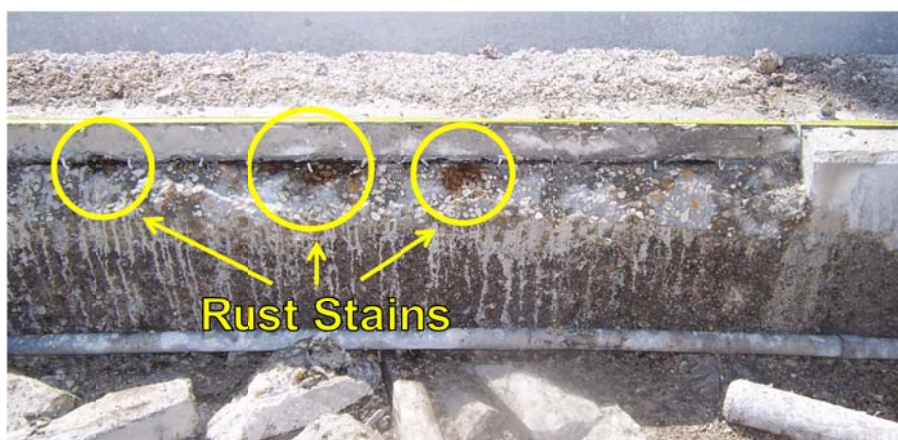
Figure 28. Exposed strand in uppermost region (nearest waterline) of autopsied pile. Note rust stains. (Photo was taken immediately after strand was exposed.)
