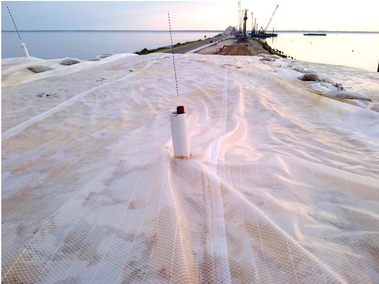
Figure 4.4. Two of four settlement rods that exhibited excessive tilting
