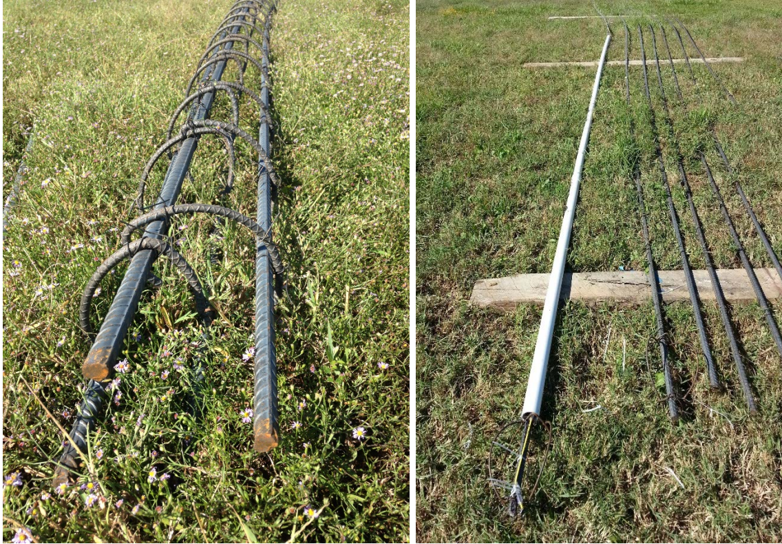
Figure 5.22. Reinforcing cage with internal hooks (left) and instrumented center bar with centralizing device and temporary protective PVC sleeve (right)
