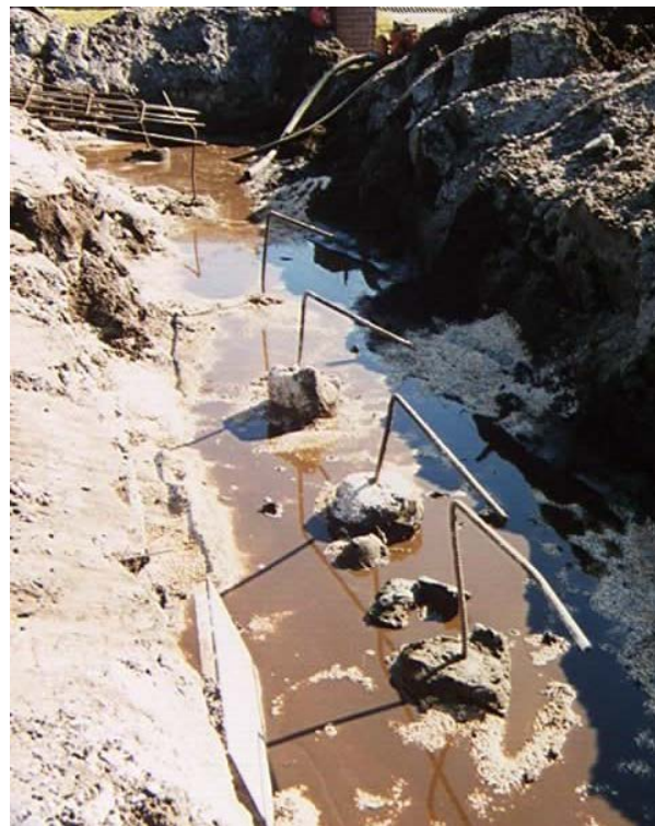
Figure 2.2. Near-surface necks in ACIP piles found upon excavation for footing
