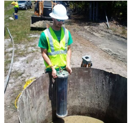
A worker prepares to lower the testing device into the slurry in a drilled shaft excavation.
