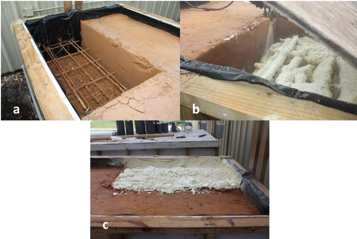
Figure 29. Filling of empty octant in box #2: a) Simulated void, b) repair using polyurethane grout, c) repaired void.
