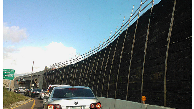
The black wall (right) is an earthwork, retained by geotextile, which supports a section of I-295 under construction.
