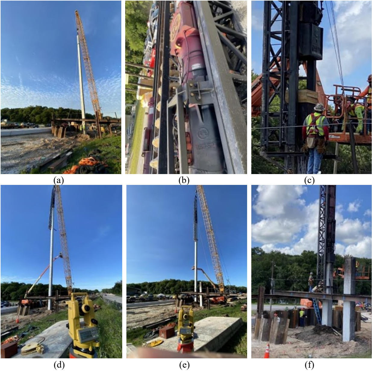
Figure 3-5. Pile driving process at Site A1: (a) hoisting of pile 13, (b) APE D50-52 used for driving piles 10 and 13, (c) installation of plywood cushion, (d) hammer in leads before pile driving of pile 13 and (e) pile 10, and (f) ending of driving.
