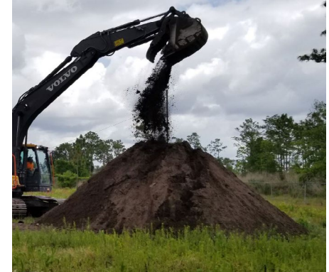
The gradual building up of a large cone of soil provides valuable data for determining soil settlement at a construction site.
