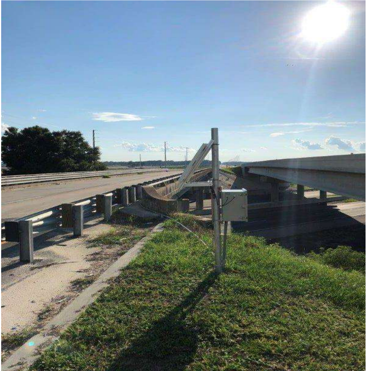
Figure 81: Solar Power Unit for Site 1 with Battery Box
