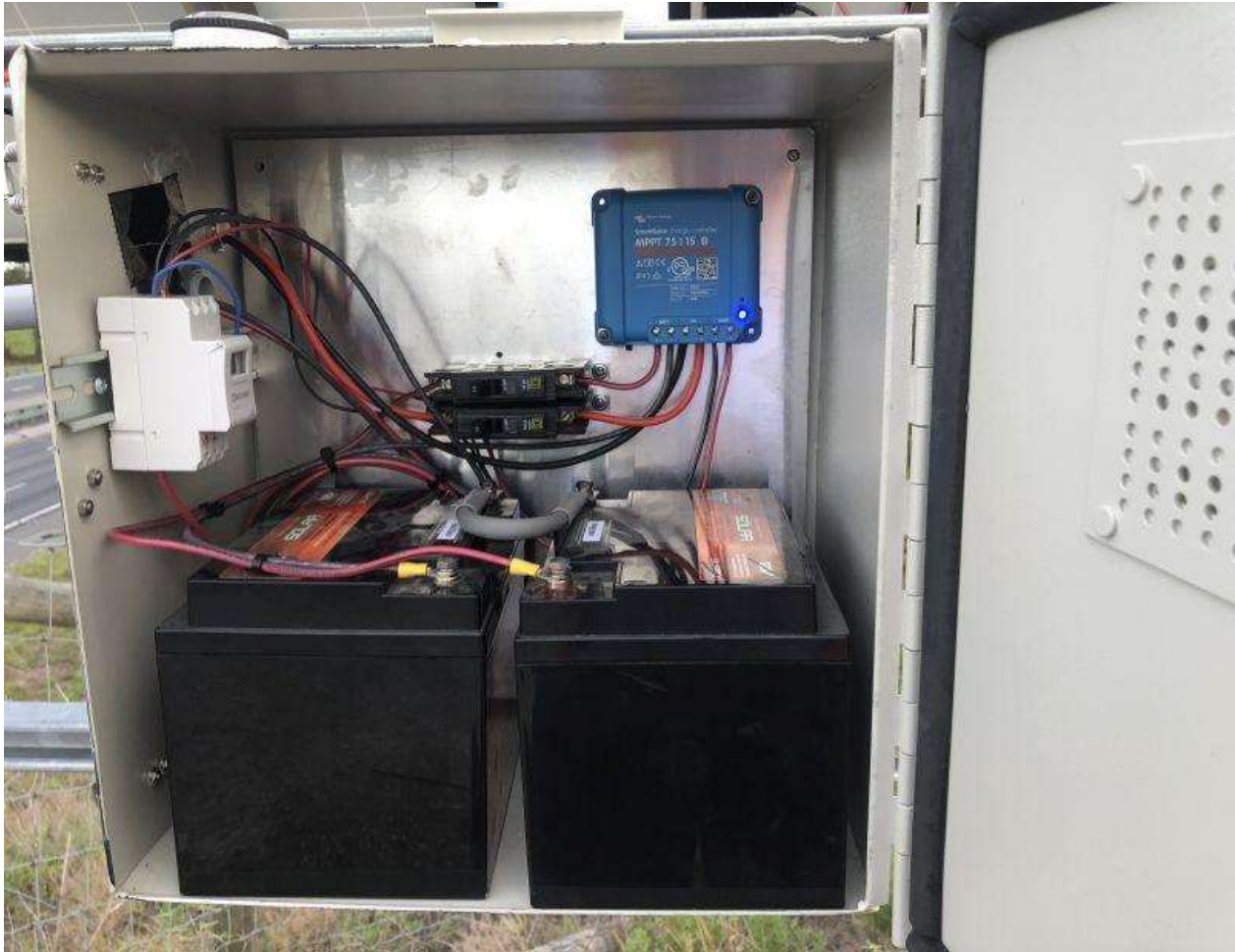
Figure 105: Batteries for Solar Panels (24V)
