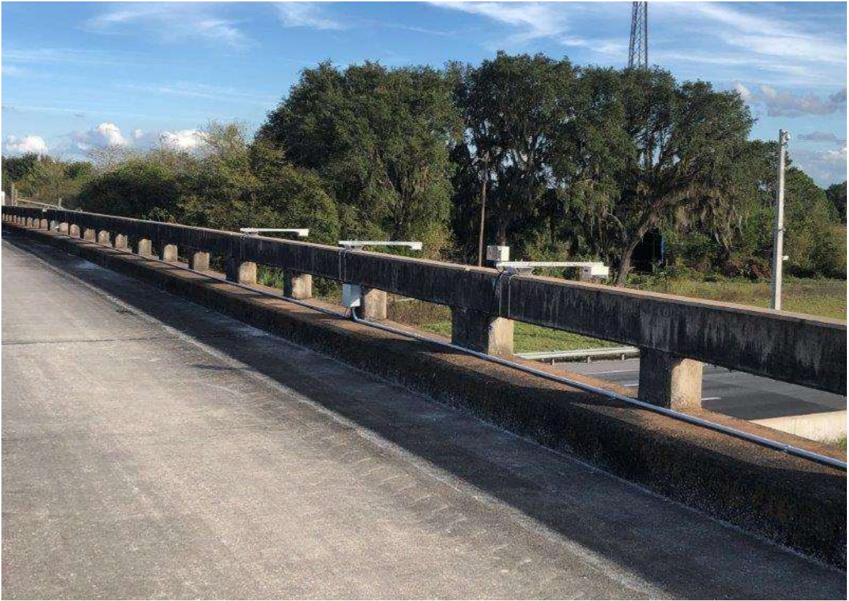
Figure 90: Capture Units on Southbound
