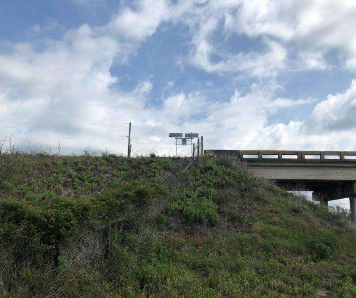
Figure 87: Solar Unit: Site 2
