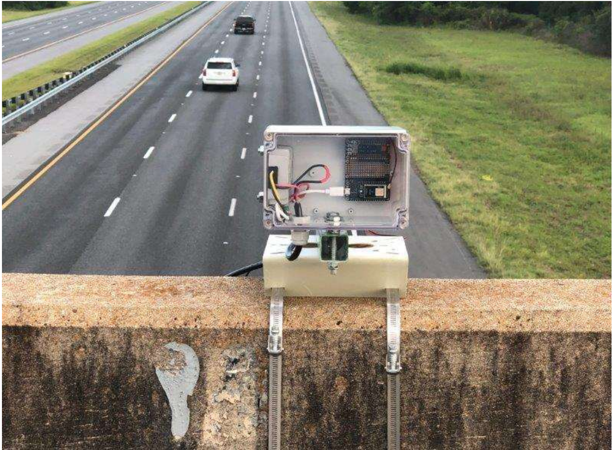
Figure 95: Site 2: Gateway Unit
