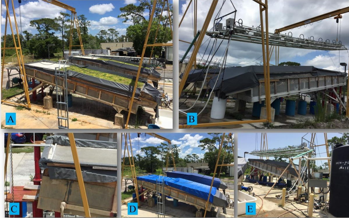
Figure 3.2. (a) Treatment and control model roadway shoulders, (b) lifted rainfall simulator, (c) roadway runoff delivered over paved section, (d) covered waterproof tarpaulin to exclude natural rainfall, and (e) water tank for supply water.
