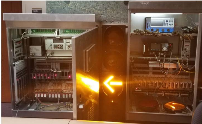
TS2 Cabinets, Different Controller Types & FYA Signal Head
