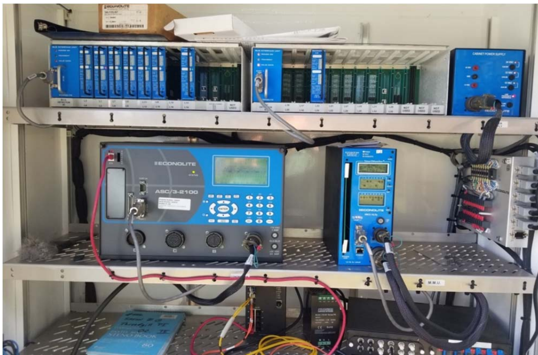
Figure 5-8: Econolite cabinet at Saxon Blvd and Threadgill Place intersection
