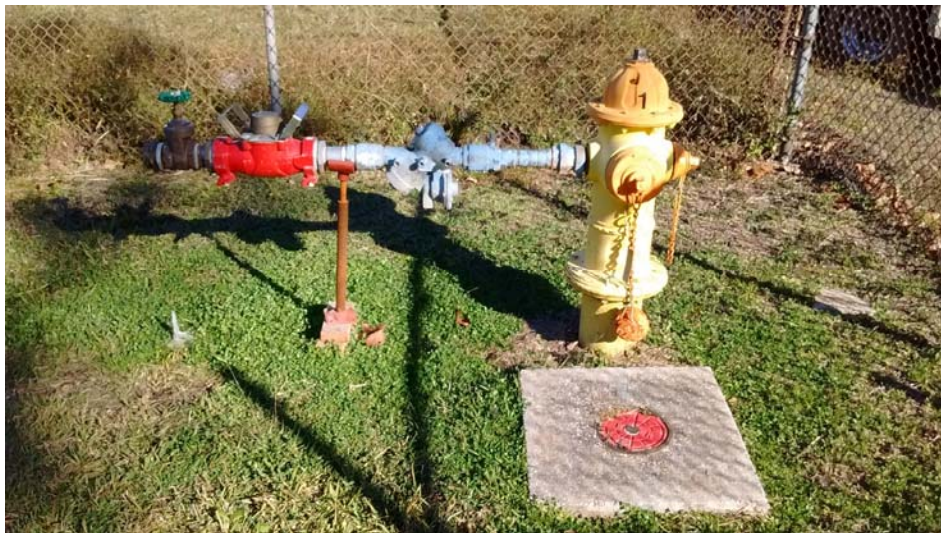
Figure 3.37. Badger meter and Watts backflow preventer installed on the fire hydrant
