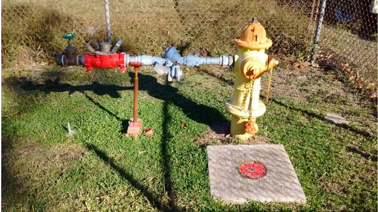
Figure 3.3: On site fire hydrant with Badger flow meter and Watts backflow prevent
