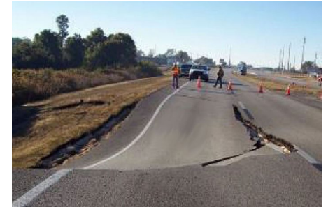
Roadway damaged by a subsidence sinkhole.
