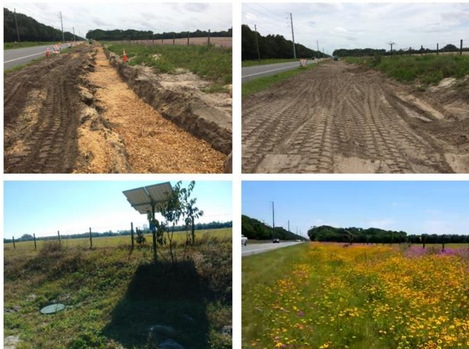
Figure 38. Construction and operation strategy in the field (upper left: construction phase; upper right: completion of construction of B&G media section; lower left: operation of pumps with solar panel in the middle of B&G media and woodchip sections; lower right: operational phase of B&G media and woodchip sections)
