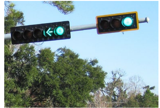
A proven safety countermeasure is the retroreflective border (right) that helps a signal stand out from its background, especially at night, dusk, and dawn.
