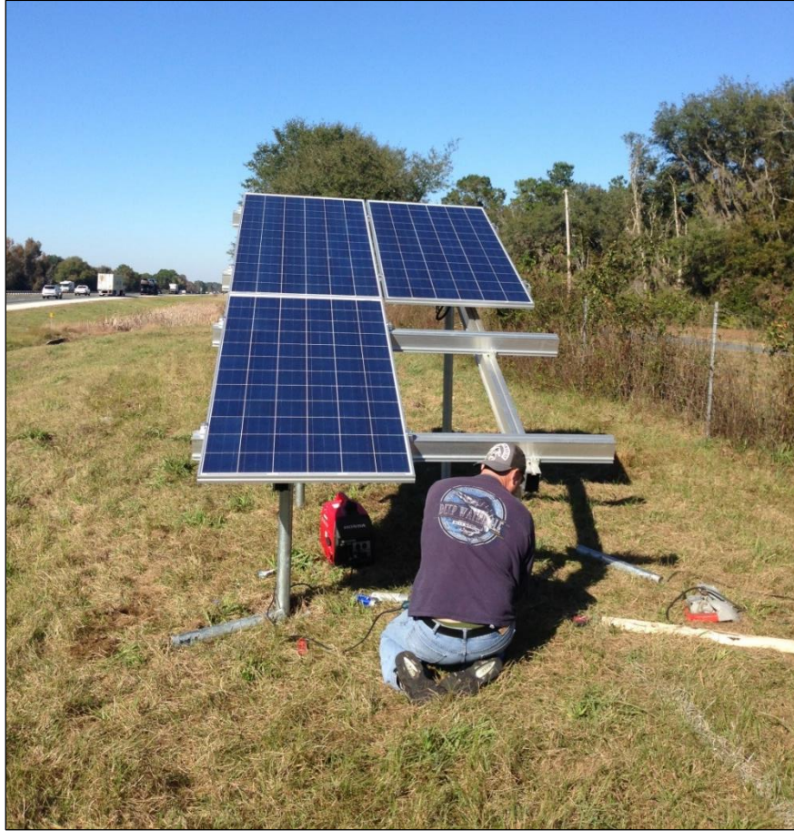
Figure 3-7: Solar Power System – Location 1
