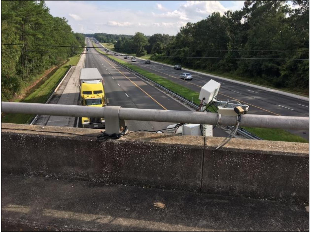
Figure B-22: Location 1 Installation1
