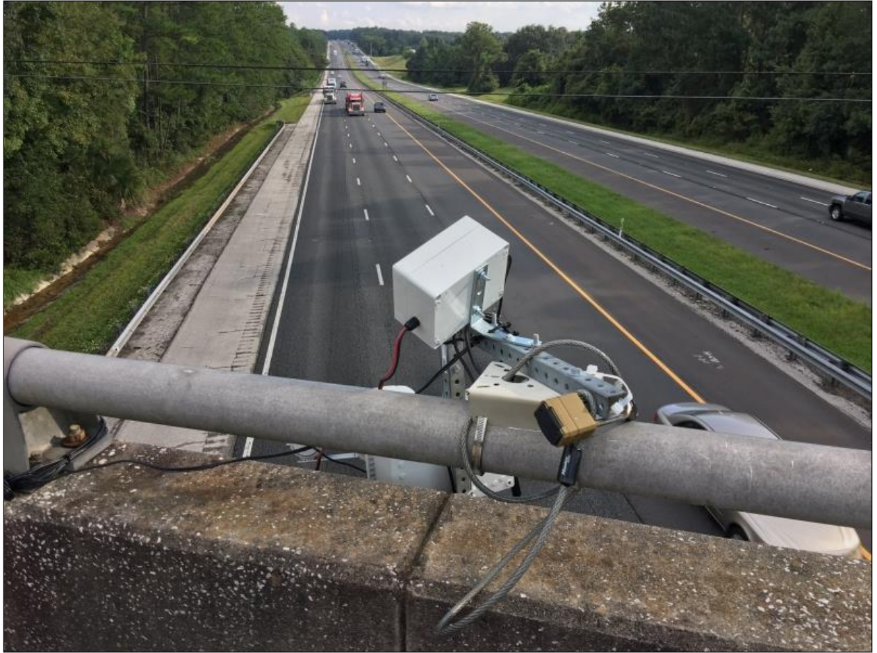
Figure B-23: Location 1 Installation-2
