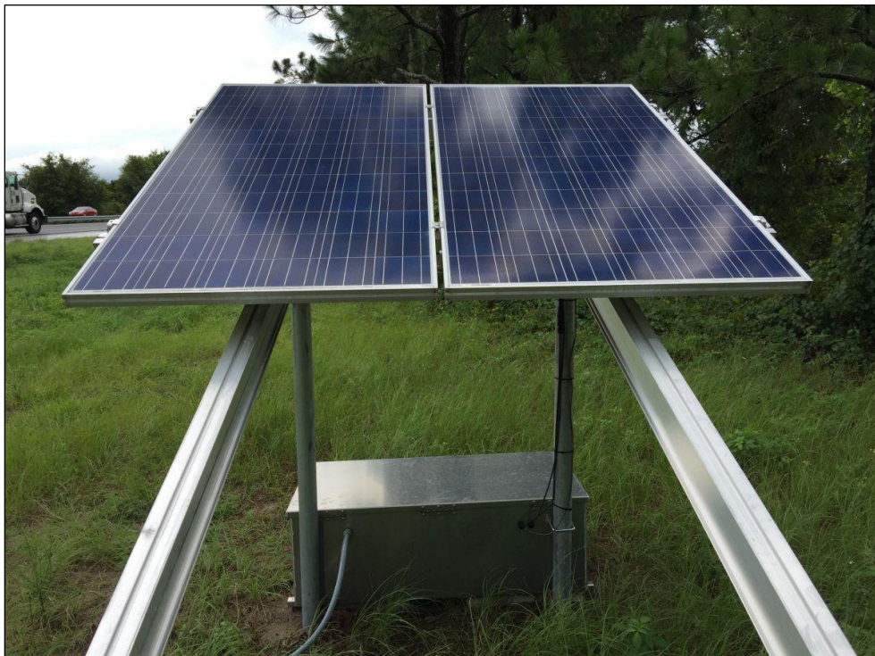
Figure B-0-12: Solar Power Unit – Location 3
