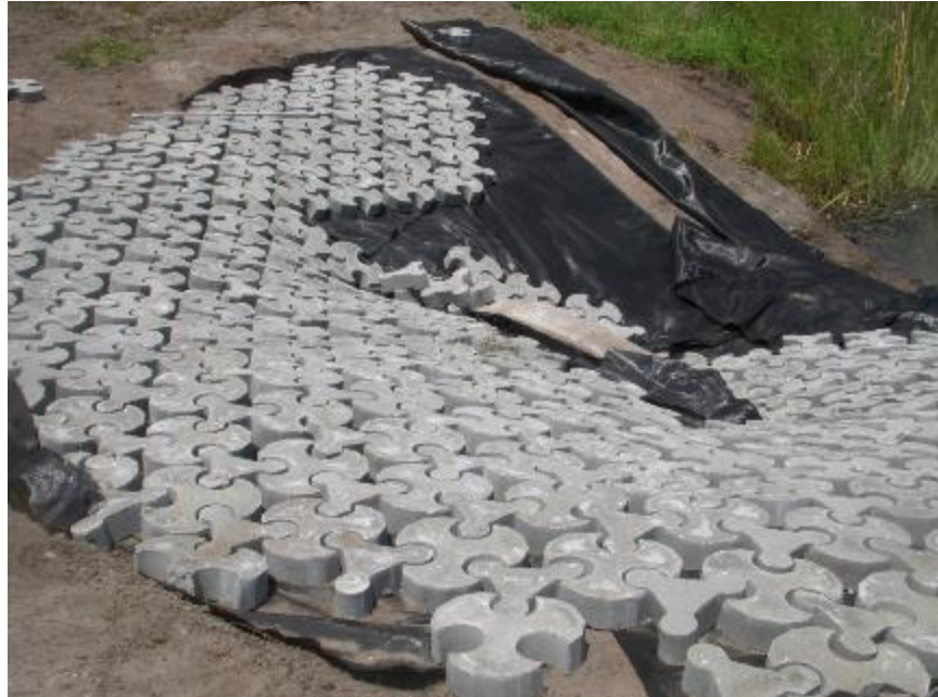
Figure 45: Tri-Lock installation around S-145 at the conclusion of the first day of work
