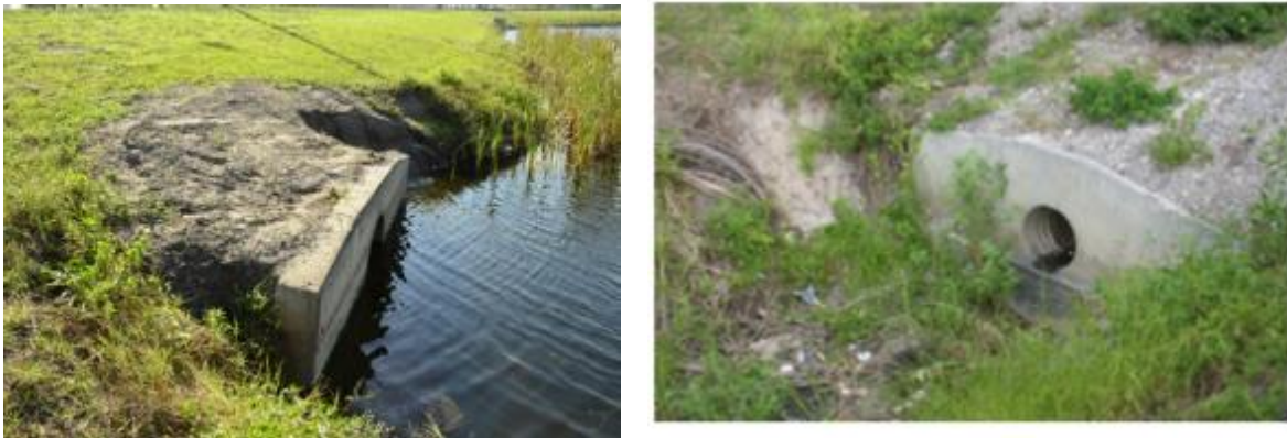
Figure 44: Pre-BMP conditions at S-139 (left) and S-145 (right), respectively
