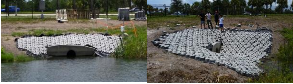
Figure 46: Tri-Lock installation at S-139 and S-145 at the conclusion of the second day of work
