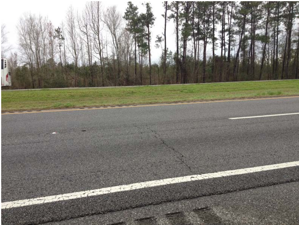
Figure 3.19 - Transverse Crack on I-10 (MP 229-230)
