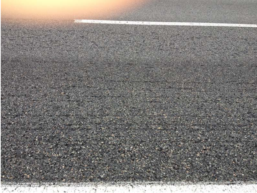
Figure 3.17 - Raveling on I-75 in Hamilton County (MP 461-462)
