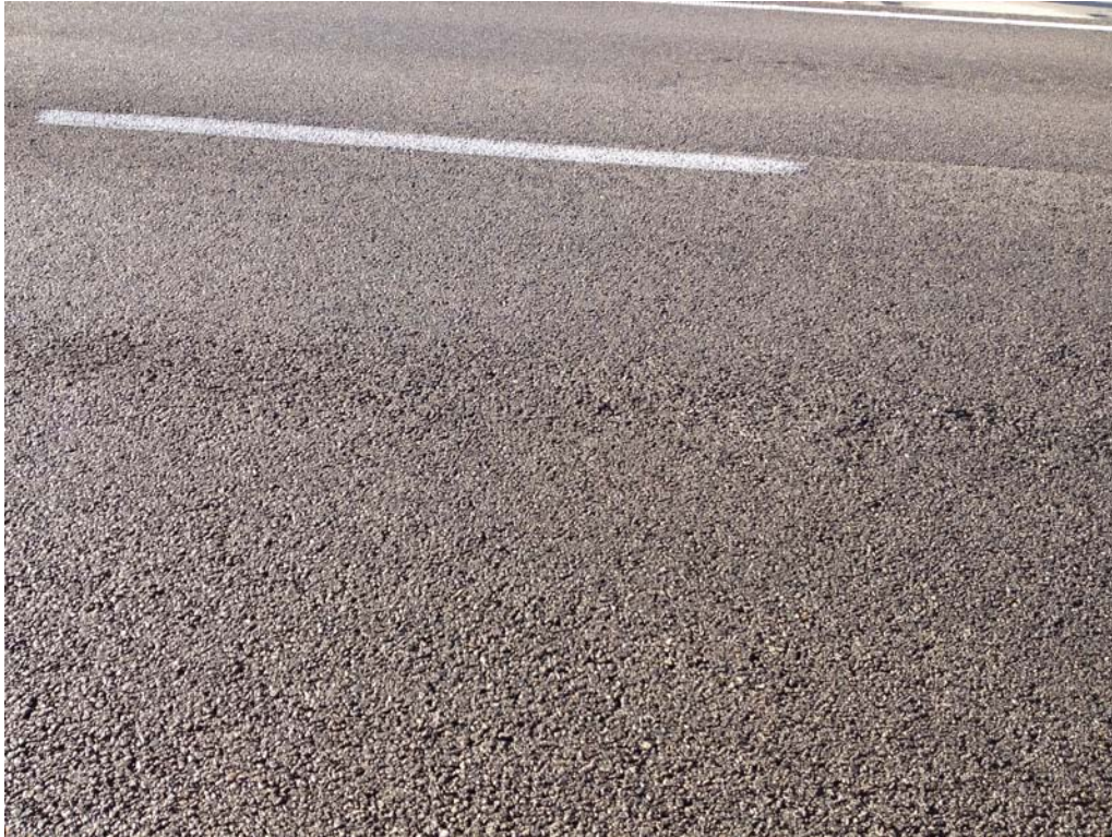
Figure 3.25 - Raveling on I-75 in Broward County near MP 30
