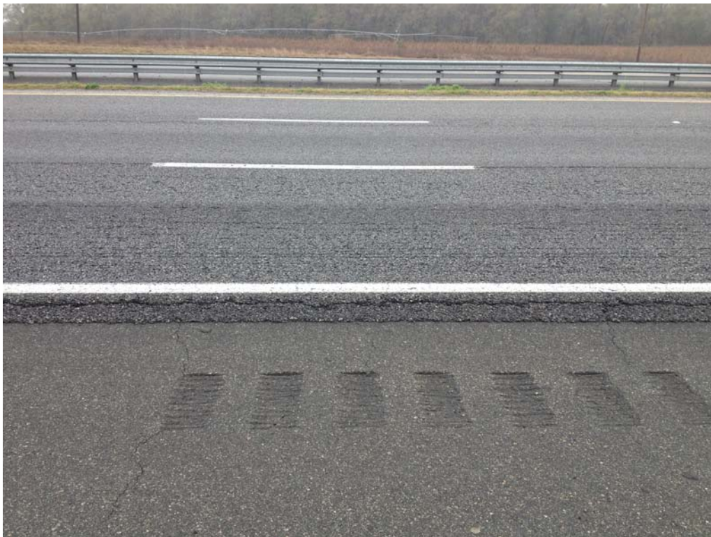
Figure 3.16 - Rutting on I-75 in Hamilton County (MP461-462)
