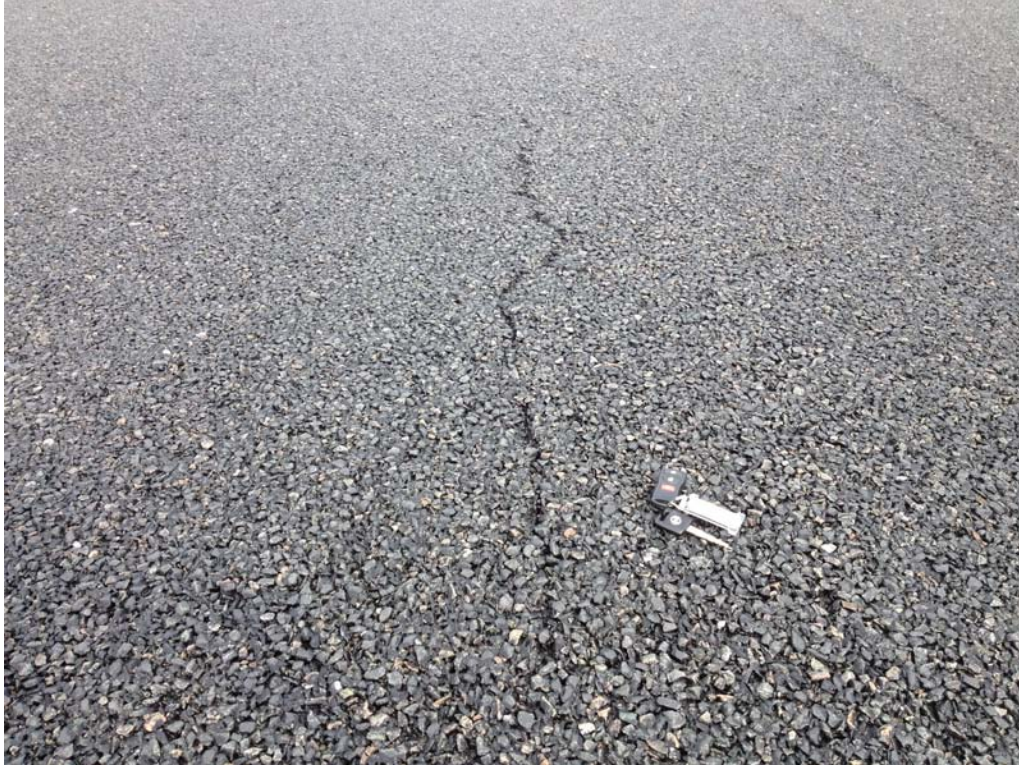
Figure 3.15 - Longitudinal Crack on SR-20
