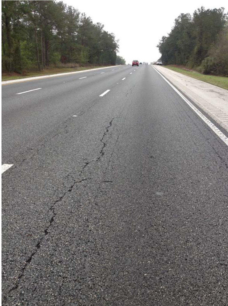
Figure 3.21 - Longitudinal Crack on I-75 in Marion County
