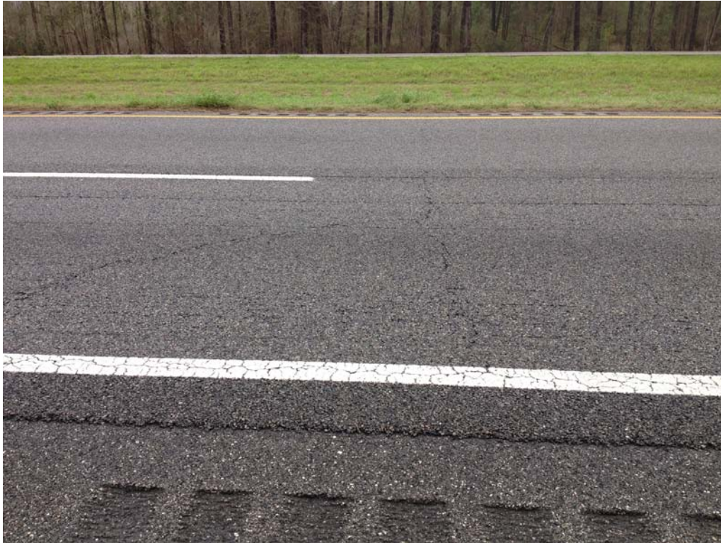
Figure 3.20 - Transverse Cracking on I-10 (MP 229-230)
