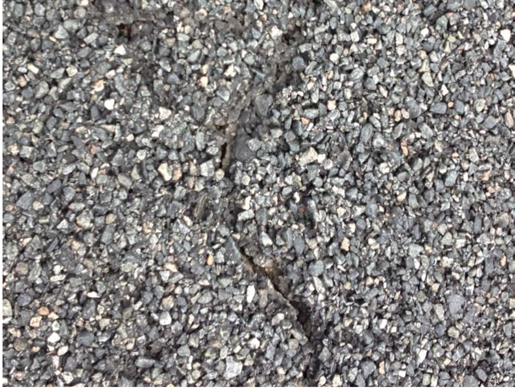
Figure 3.22 - Close-up of Longitudinal Crack on I-75 in Marion County
