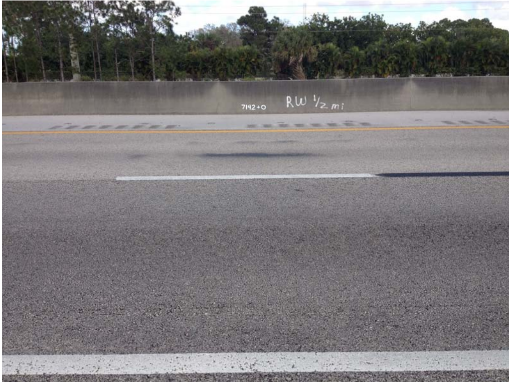
Figure 3.24 - Flushed Area on Florida Turnpike near MP 133
