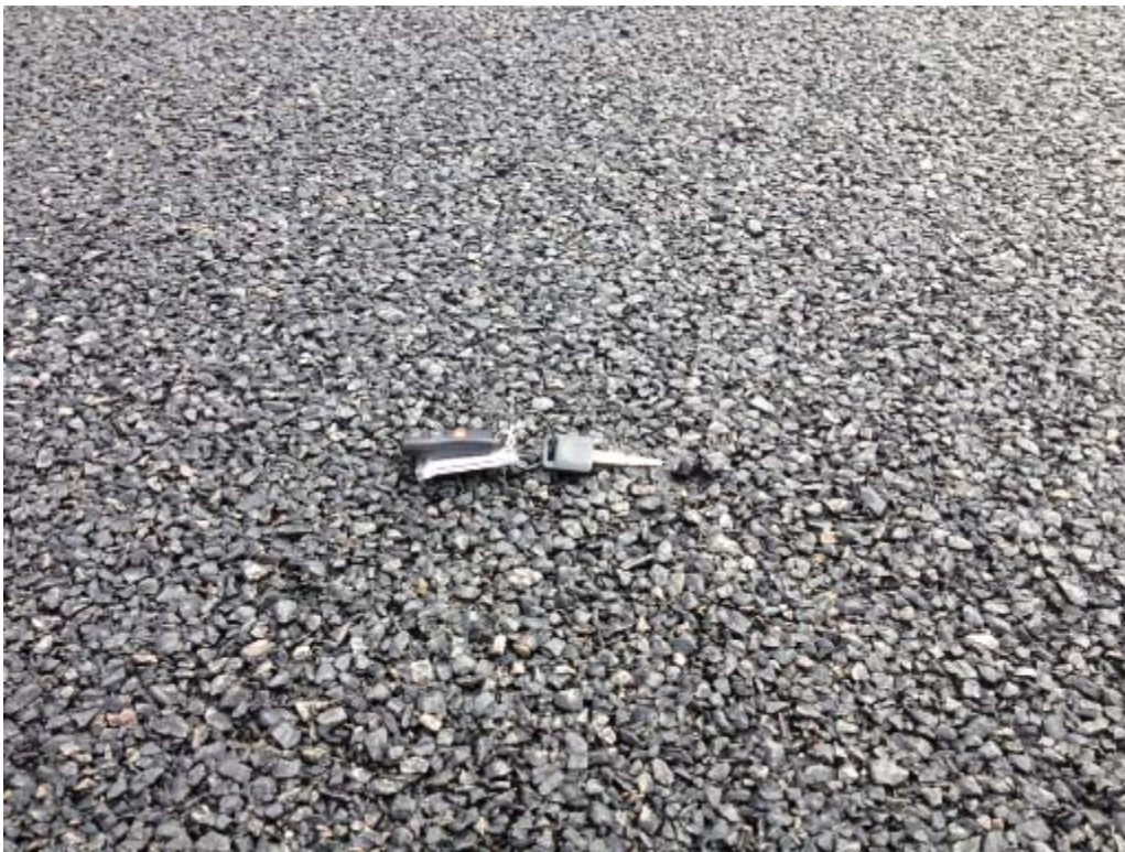
Figure 3.14 - Aggregate Pop-out on SR-20
