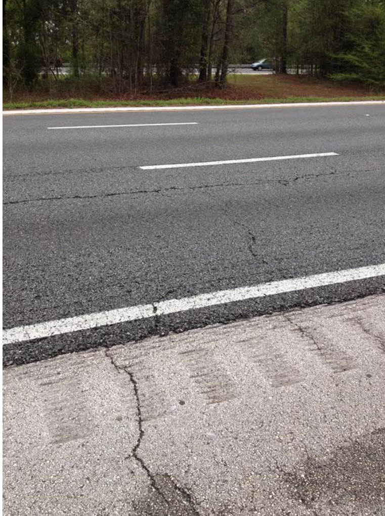
Figure 3.23 - Transverse Crack on I-75 in Marion County
