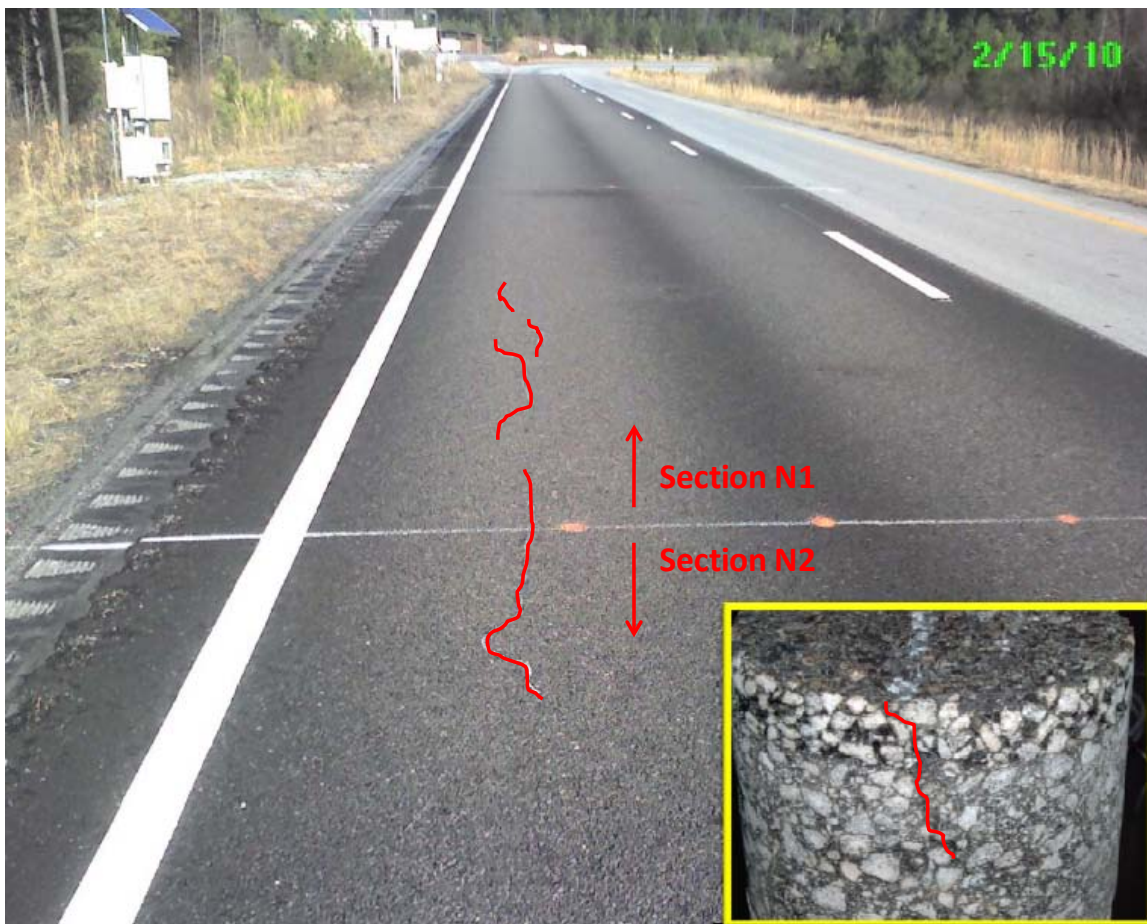
Figure 1.1 - Top-down Cracking at the NCAT Test Track for FDOT's FC-5 Mixtures
