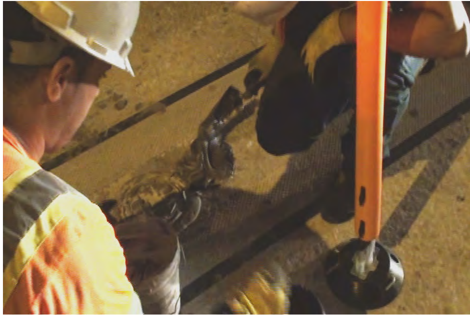
Figure 5. Epoxy Failure and Pavement Failure Replacement.
