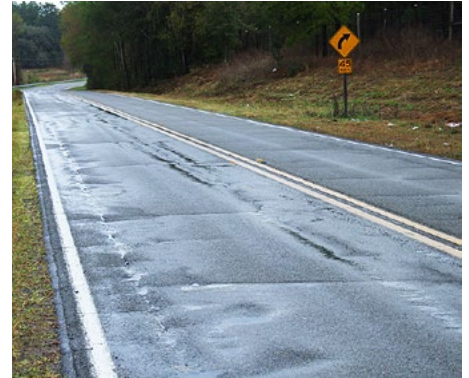
Damage to the road surface can allow water to gather, creating an unsafe condition.
