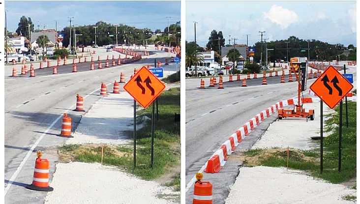
This image from this project's field tests compares the use of drums (left) and LCDs (right) to mark the same business entrance.
