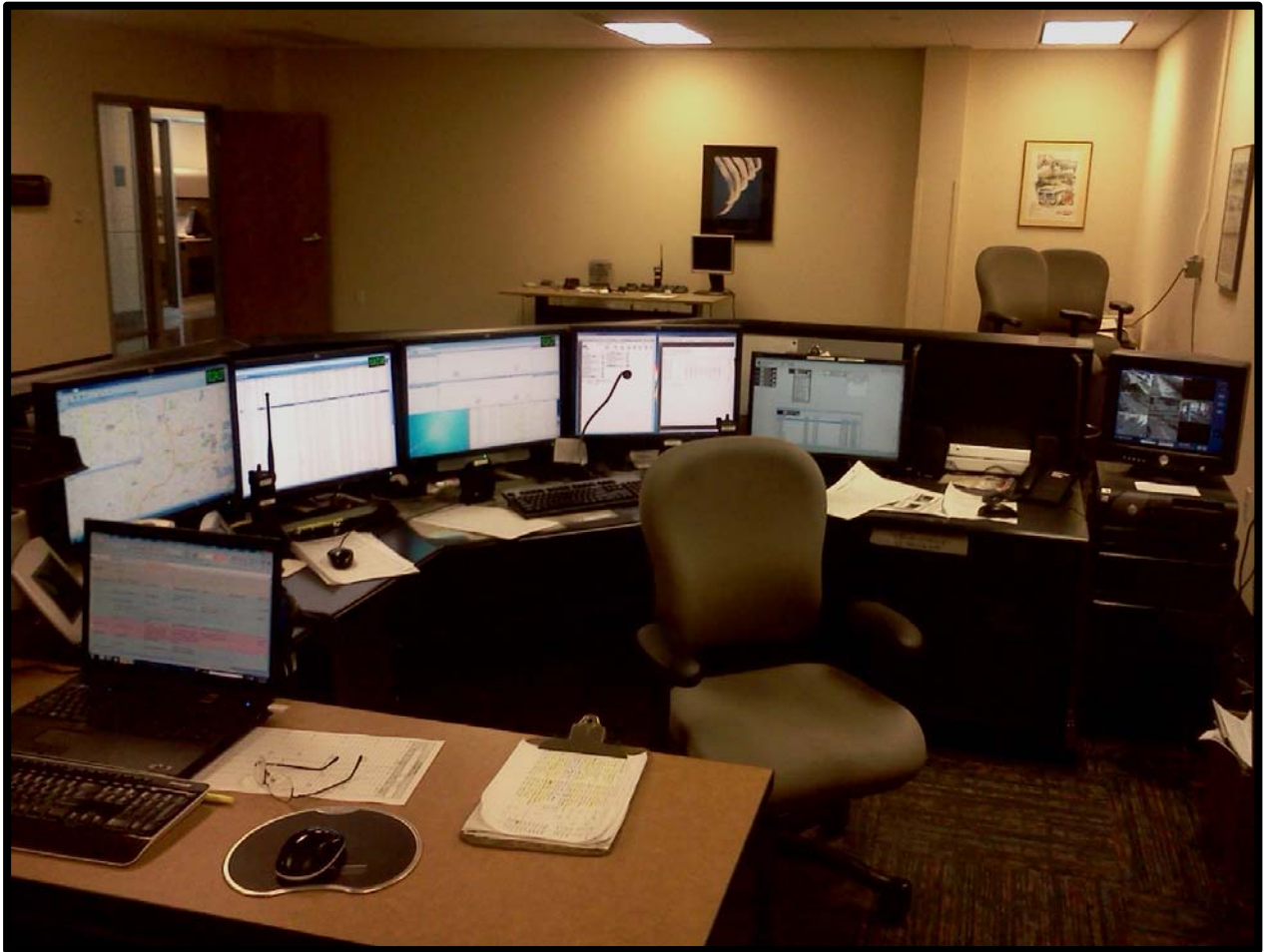
Figure 3-2 Radio Control Room – South County Station
