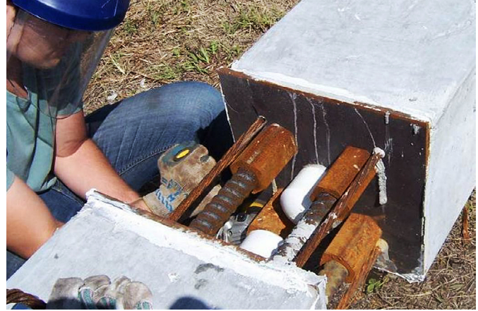
A worker puts the finishing touches on a test pile. The ducts containing the steel strand are visible here by the white caps that seal them.
