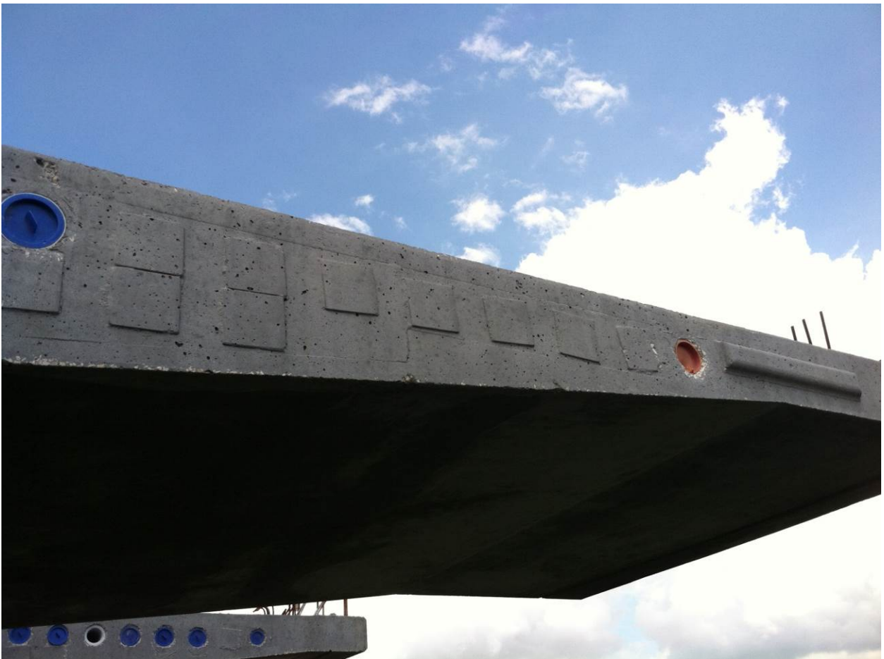
Figure A6 PT strand (left) and PT bar ducts (right) with temporary end caps in casting yard (14U, used for PT bar duct RH record). Note uncapped duct in nearby segment. No picture for 13U
