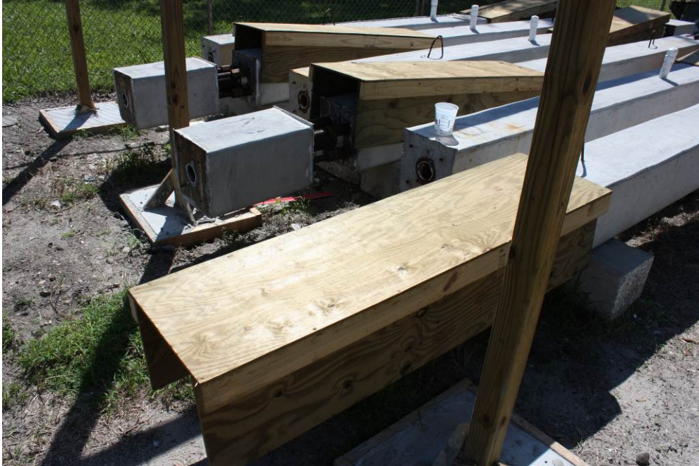
Figure 17 Wooden End Cowls at USF Facility
