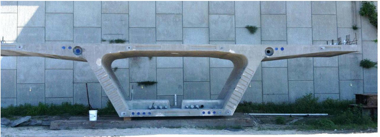
Figure A1 Typical box girder segment resting on ground beneath span 10-11 Note some ducts left uncapped. No RH probes were placed in this segment, pictured only for overall appearance information
