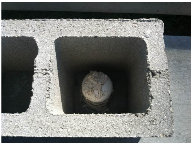
Figure 20 RH Access Port Cinder Block Covers, without Lid
