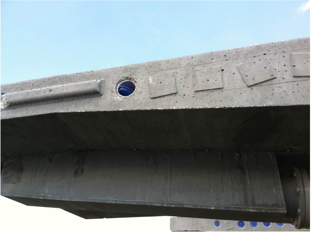
Figure A7 Uncapped PT strand duct in casting yard segment (14U, no probes placed in this duct)
