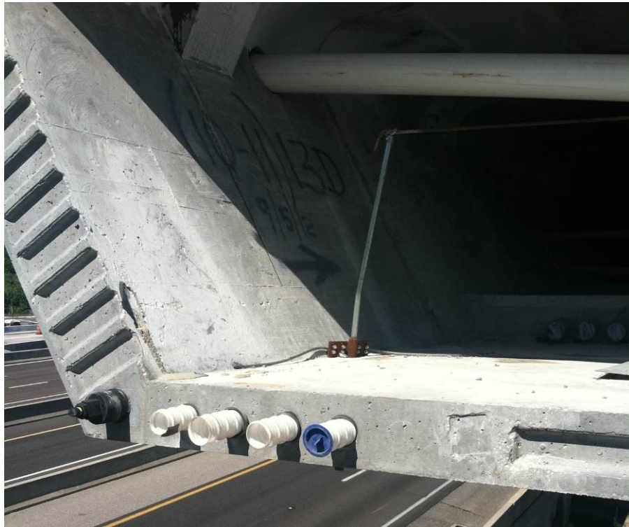
Figure A5 Uncapped PT strand ducts in partially constructed span (10-11). Probes not placed in this segment
