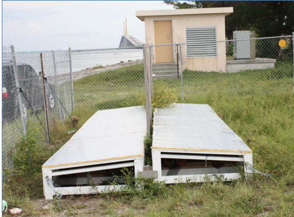
Figure C2 SSK Duct Facility in the Closed Position - Sunshine Skyway Bridge Main Span and Generator Control Room in the Background
