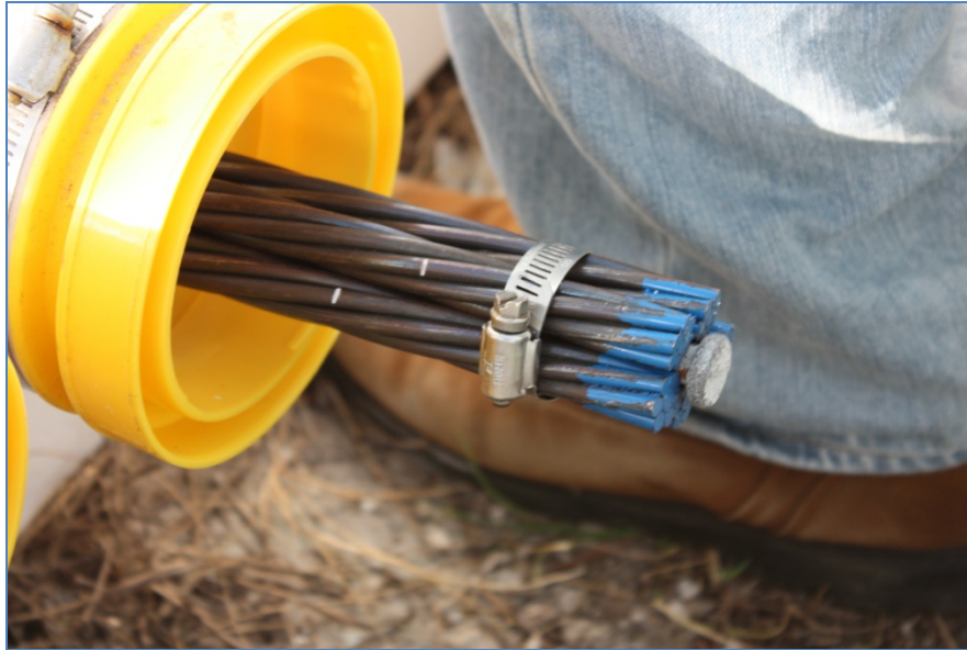
Figure C5 Strand Group Ready for Duct Insertion with Galvanized Spike Secured with Stainless Steel Hose Clamp
