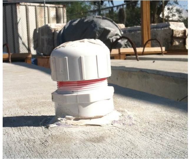
Figure 19 RH Probe Access Port Tube after Height Reduction
