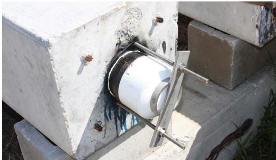
Figure 16 Custom End Cap installed on East End of Duct 6 at USF Facility
