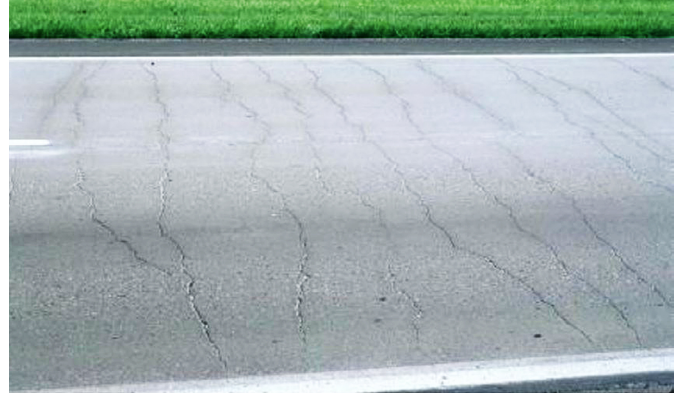
The stretch of concrete pavement shows the effects of thermal cracking.
