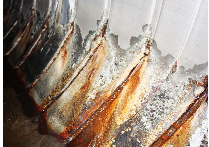
Extensive corrosion and mechanical damage are evident in this SRAP set in limestone backfill.
