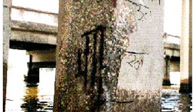
Severe corrosion damage to reinforcing steel in this column has caused the overlying concrete to spall.
