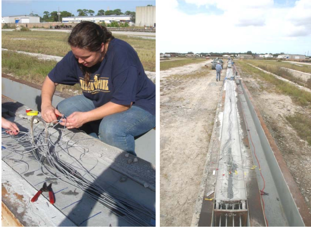
Figure 5.23 Surface gage wiring back to data collection systems.
