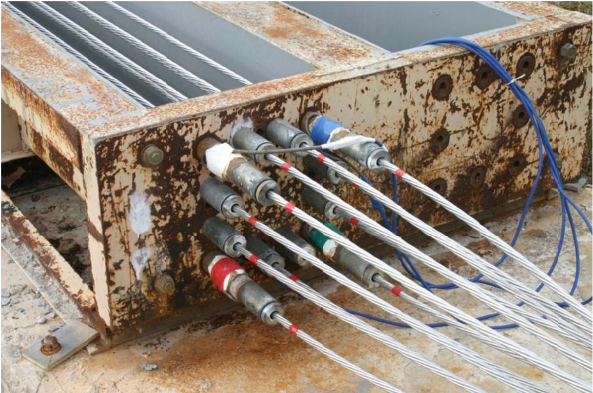
Figure 5.10 Load cells inserted between chucks and bed header plates.
