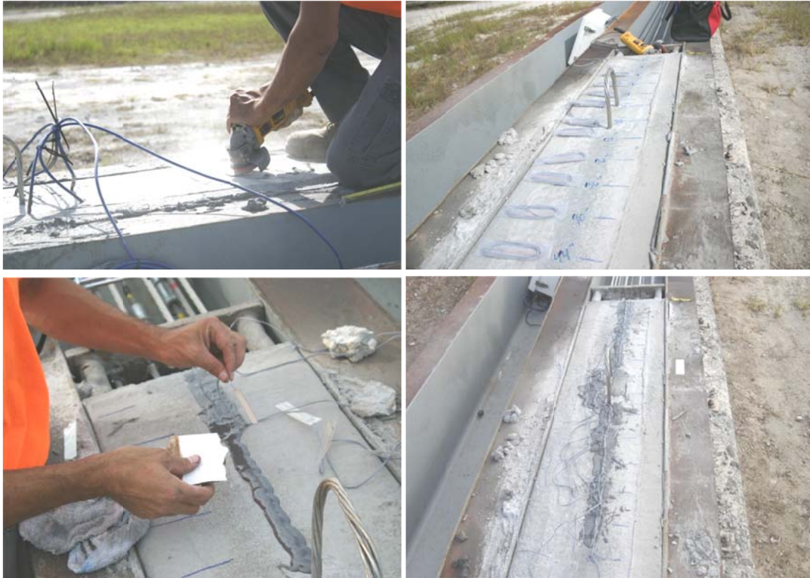
Figure 5.22 Grinding pile (top left); gage layout (top right); embedding gages in epoxy (bot left); and finished instrumentation (bot right).
