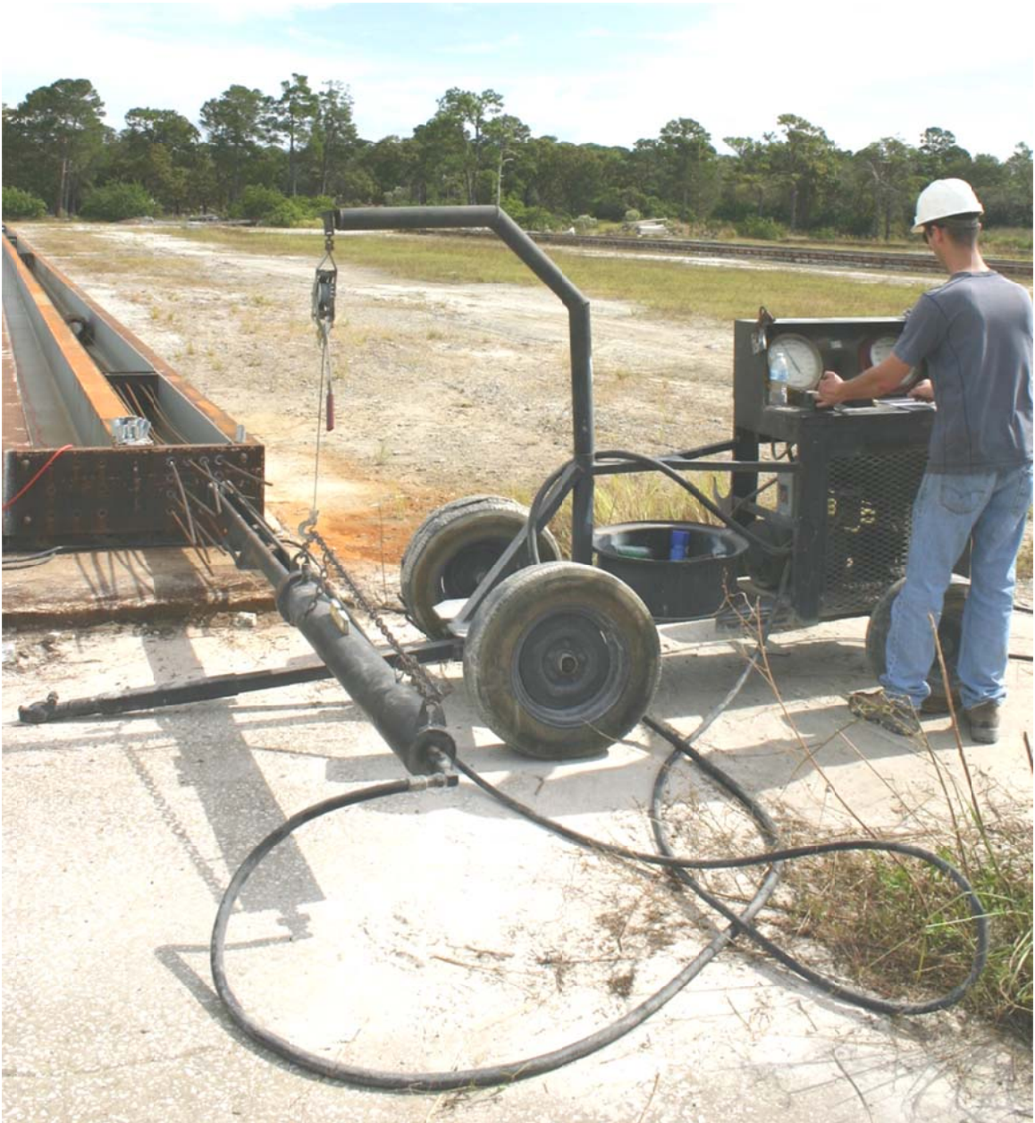
Figure 5.13 48in stroke hydraulic jack used to cycle and bring strands to design load.
