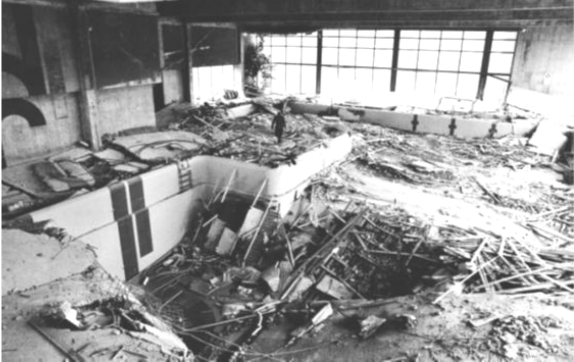
Figure 2.4 Suspended ceiling collapse of Uster swimming pool caused by transcrystalline stress corrosion cracking (Faller, 2003).
