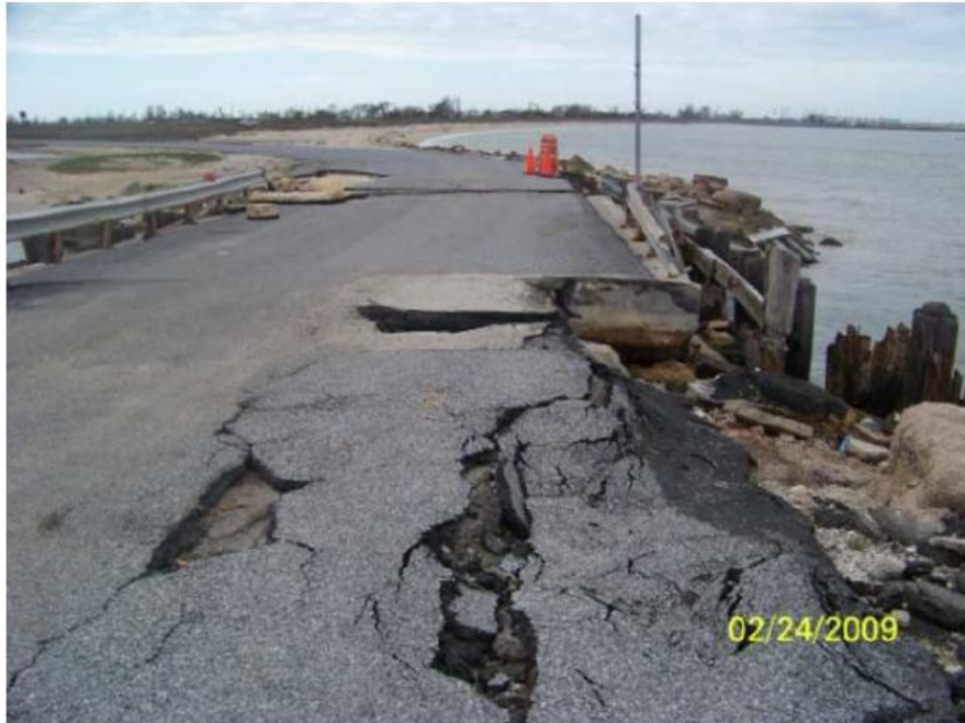
Figure 2.1. Bridge approach undermined by scour due to Hurricane Ike (Stearns and Padgett, 2011)
