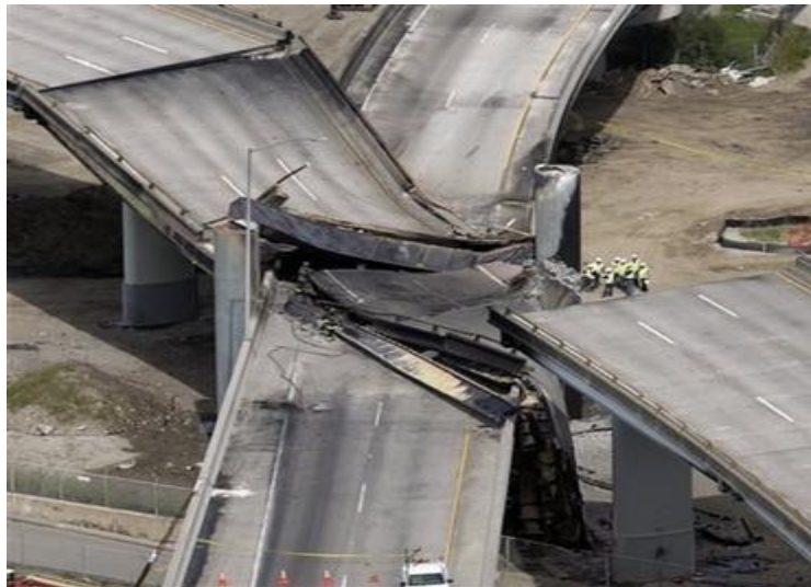
Figure 7.19. San Francisco Oakland Bay Bridge after fire damage
