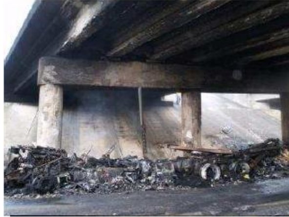
Figure 7.18. Detailed display of damage to the bridge elements (Lessard 2010)
