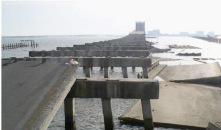
Figure 2.5. US-90 Biloxi-Ocean Springs Bridge showing the primary mode of failure in severely damaged bridges: span unseating due to storm surge-induced loading (Padgett et al., 2008)
