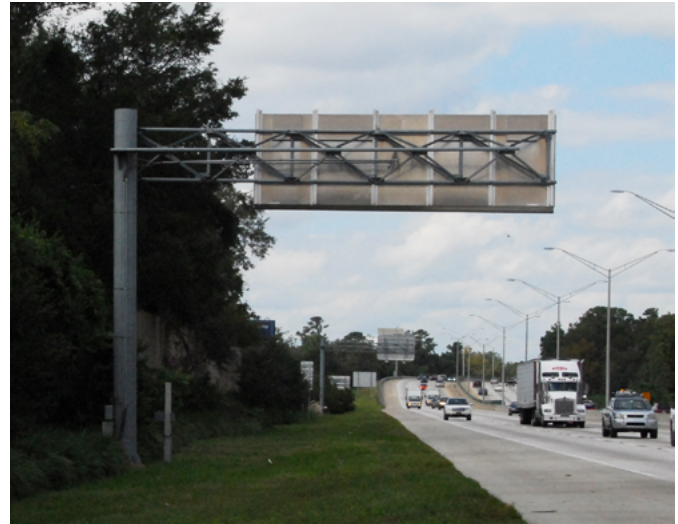
Fiber-reinforced polymers offer advantages over steel in applications such as some components of this cantilever sign on I-95.
