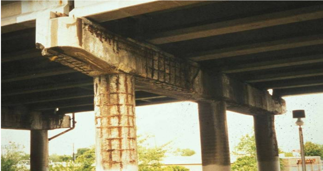
Figure 2.4: Concrete structure deteriorated by the corrosion of steel reinforcement
