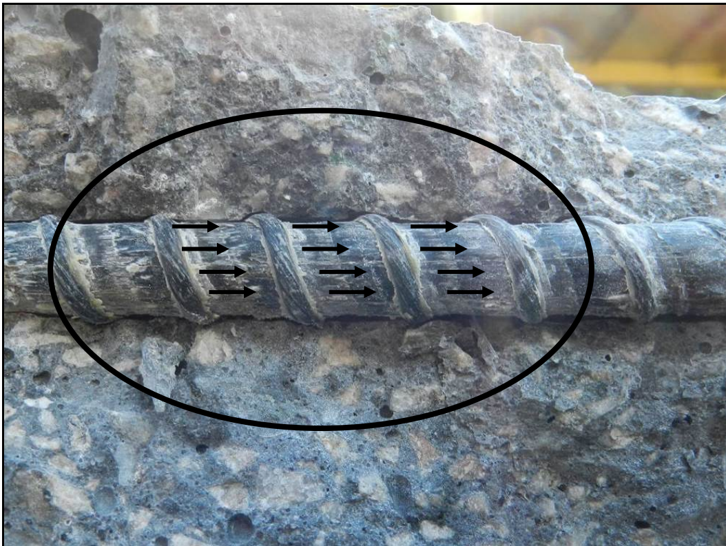
Figure 5.233: Exposed BFRP bar with debonded spiral wrapping
