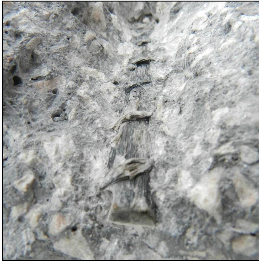
Figure 5.234: End of a tested specimen with concrete cover removed
