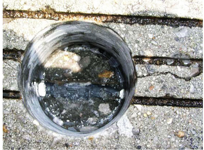
The development of a transverse deck crack, at the right, is examined by taking a core sample.
