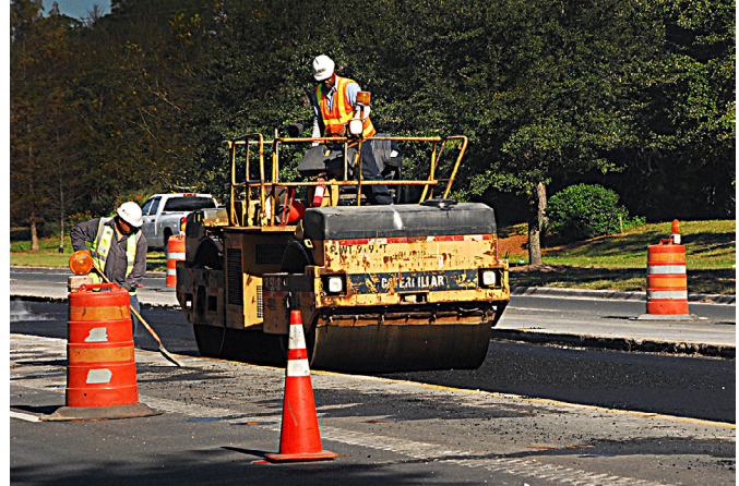
Vibratory compactors and pile drivers produce intense vibrations that can damage susceptible structures or sensitive equipment.
