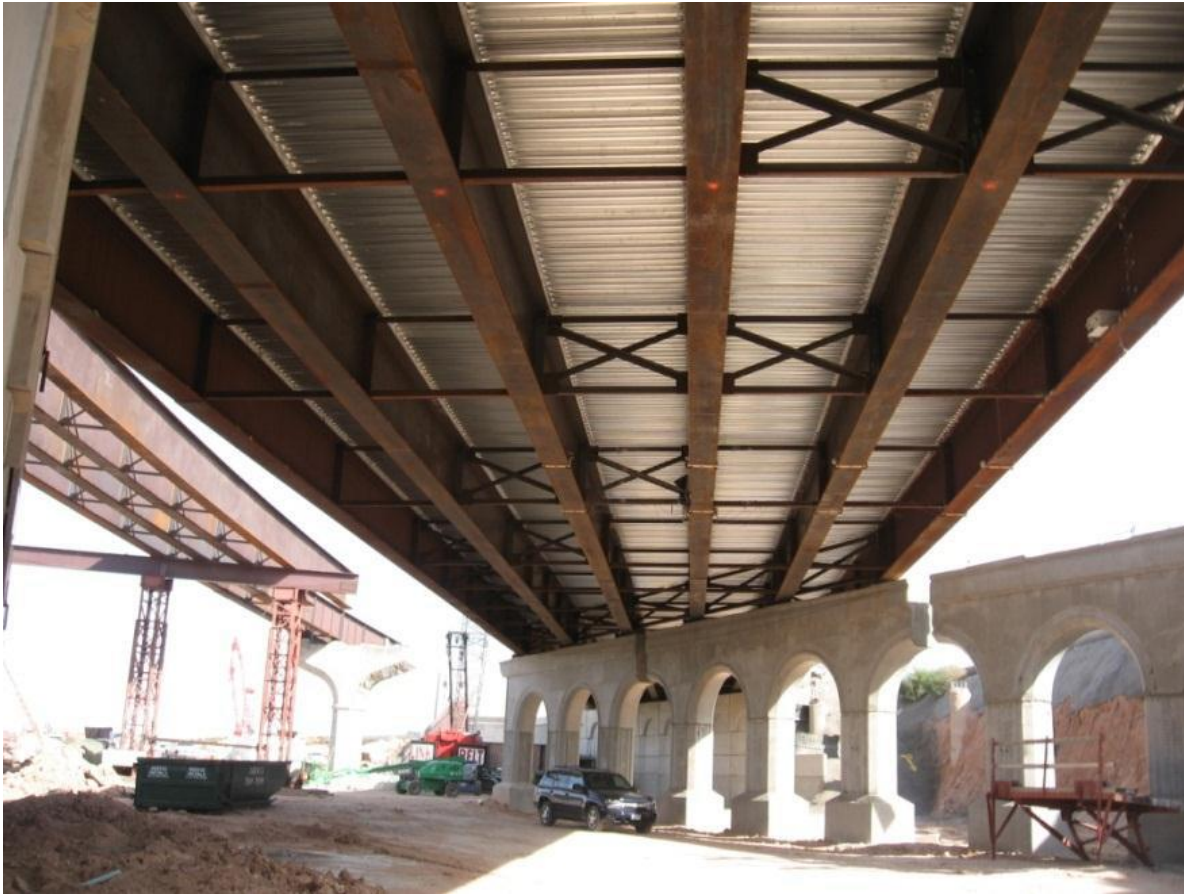
Figure 5.20: Lean-on bracing system in 19 th street Bridge
