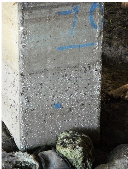
Wet-dry cycling speeds the effect of sulfate and pH, as shown by the heavily etched region of this piling installed in 2009.
