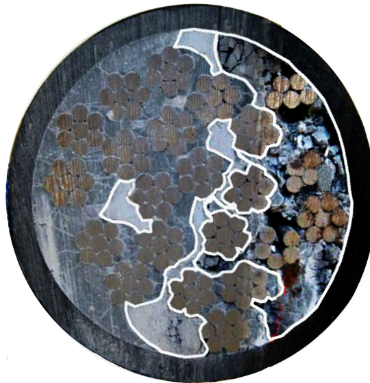
In this cross-section of a post-tensioning duct, clusters of tensioning strands can be seen scattered throughout, surrounded by grout. Grout condition varies from intact (left), to decaying (outlined gray areas; middle), to decayed (right), where voids and corroded tendons are visible.
