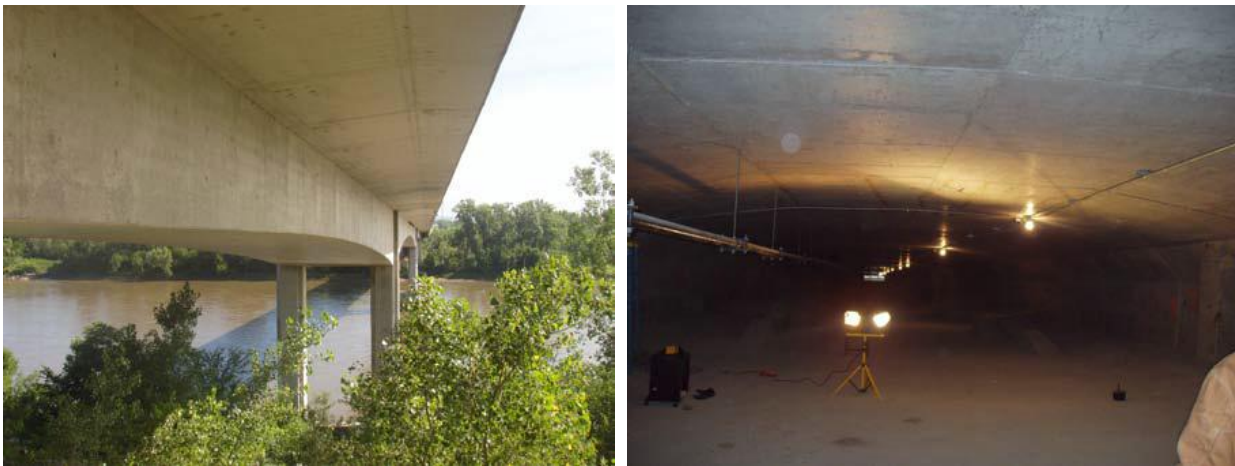
Figure A.7: An example of major segmental post-tensioned bridge inspected by P.I.
