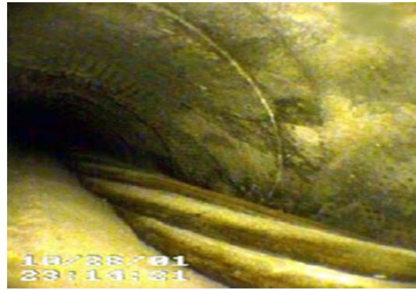
Partially grouted duct with partially exposed strands
