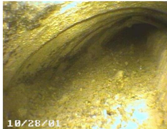
Partially grouted duct but no strand exposure
