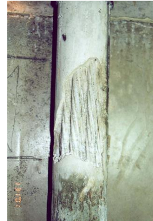
(b): Lack of corrosion activity in the voided area
