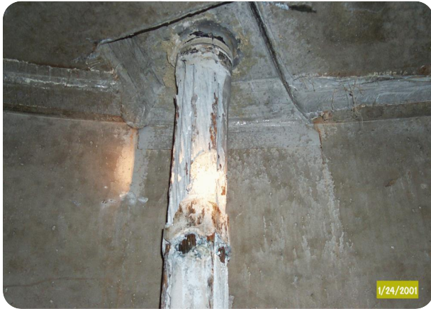
(a): Corrosion activity in the voided area
