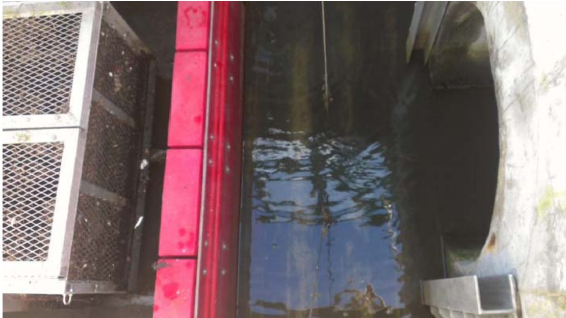
Figure 6-9 Actual Operation of On-Line Sorption Filter during Low Flow
