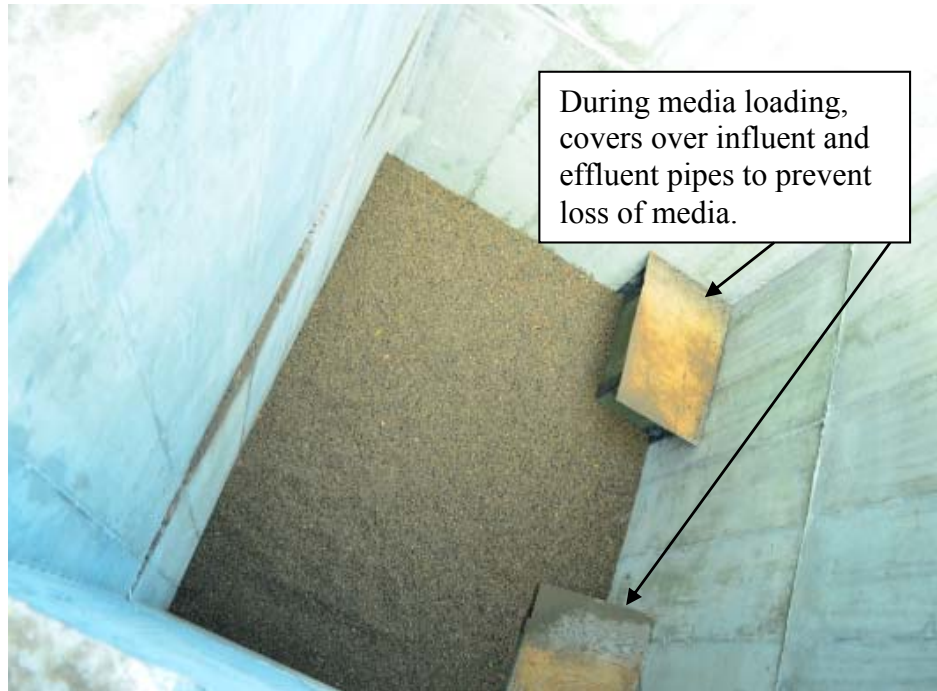
Figure 6-6 Up-flow Off-Line Sorption Filter after Media Placement
