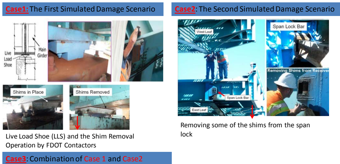
Figure 31 -Implemented damage scenarios on the Sunrise Bridge
