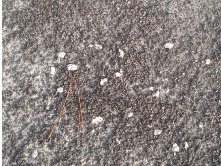
Figure 19: Number 57 stones that were embedded into surface of porous asphalt after driving over by vehicles
