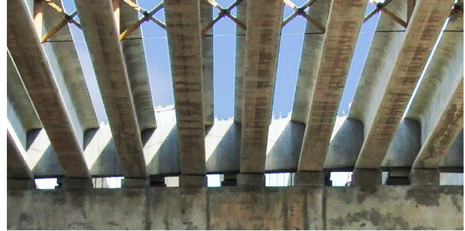
The cross-braces between these girders stabilize them against loading from the wind and the construction activities that will take place on top of them.
