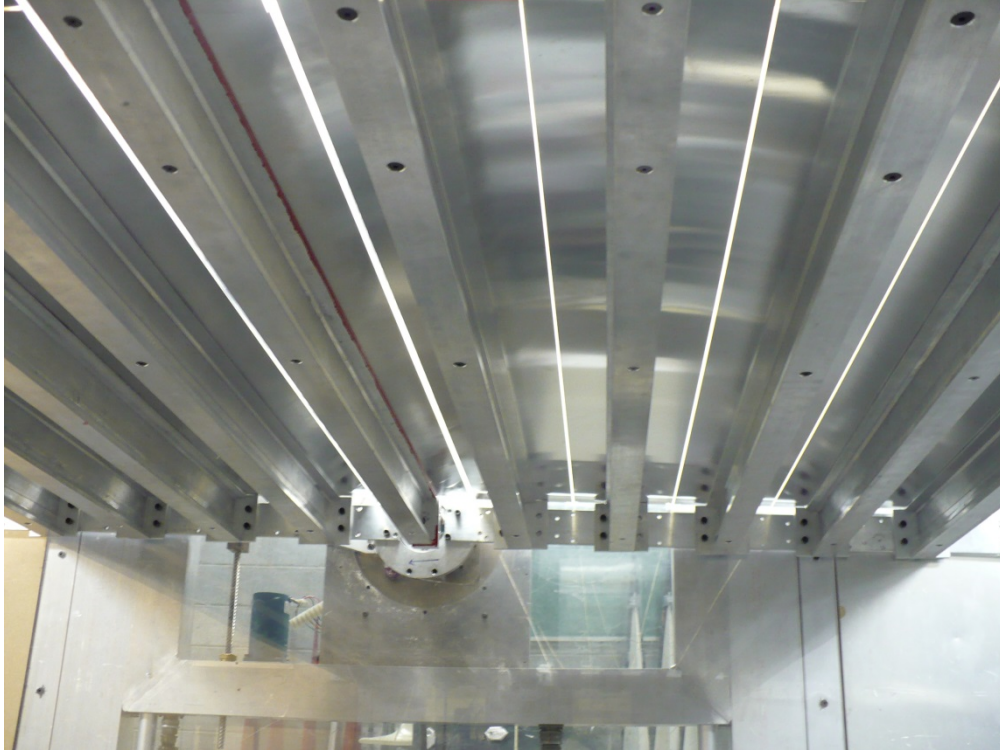
c) INSTRUMENTED GIRDER AT 5 th POSITION
