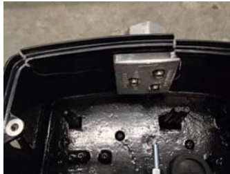
Figure 4-5. Reinforced disconnect box failure mode, flexure
