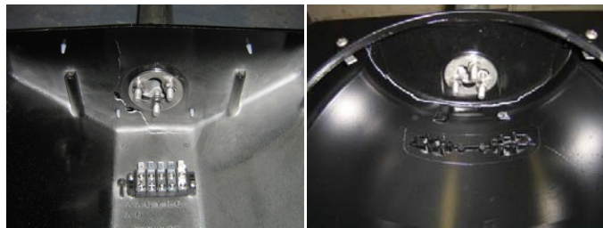
Figure 4-4. Signal head failure modes, tension
