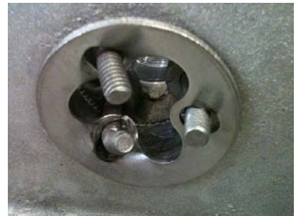
Figure A-16. DL2.3 failure mode, attachment hardware
