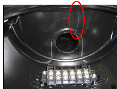
Figure A-36. SH4.3 failure mode, crack at top connection
