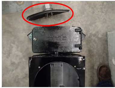
Figure A-39. C1.2 failure mode, crack around top of disconnect
