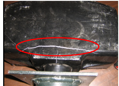
Figure A-60. DS1.3 failure mode, crack around bottom
