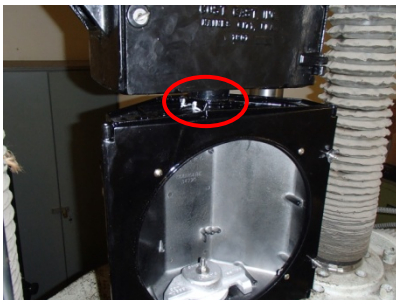
Figure A-94. C1.1 failure mode, crack at top of signal
