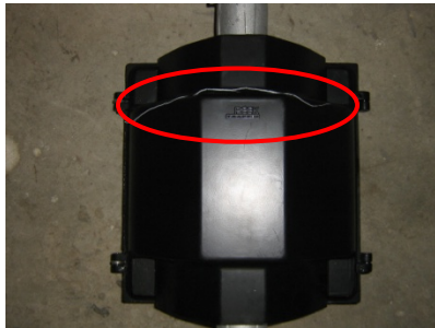
Figure A-82. SH2.1 failure mode, crack around back of signal
