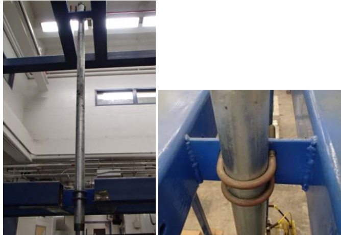
Figure 3-2. Pipe hanger connection (photos courtesy of author)
