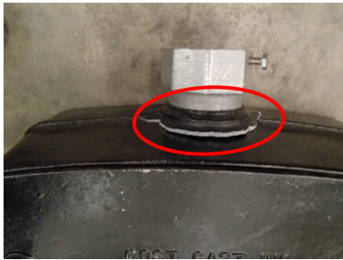
Figure A-38. C1.1 failure mode, crack at top of disconnect
